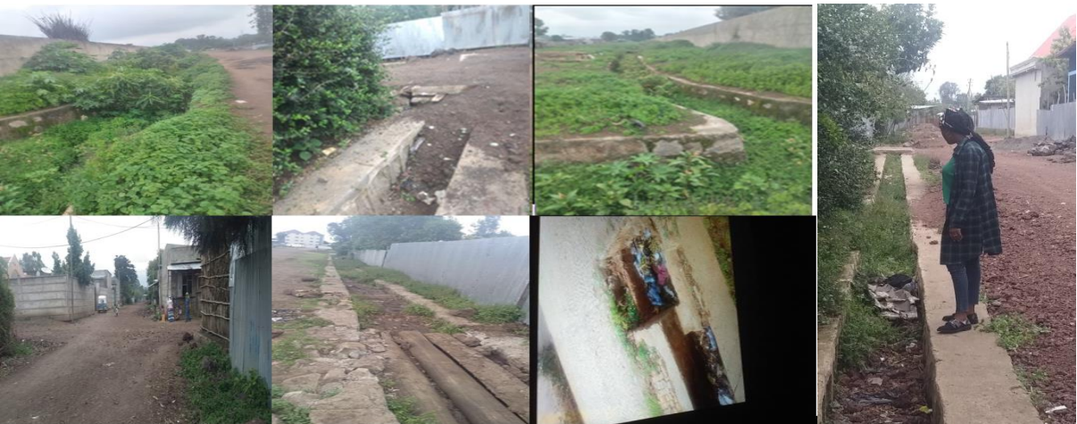
Figure 2: Drainage lines filled by grass, sediment and have no road drainage structure on both sides (site visiting time)
