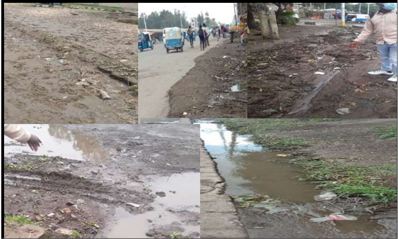
Figure 4. 2: Lack of inadequate slope cause siltation and ponding.
