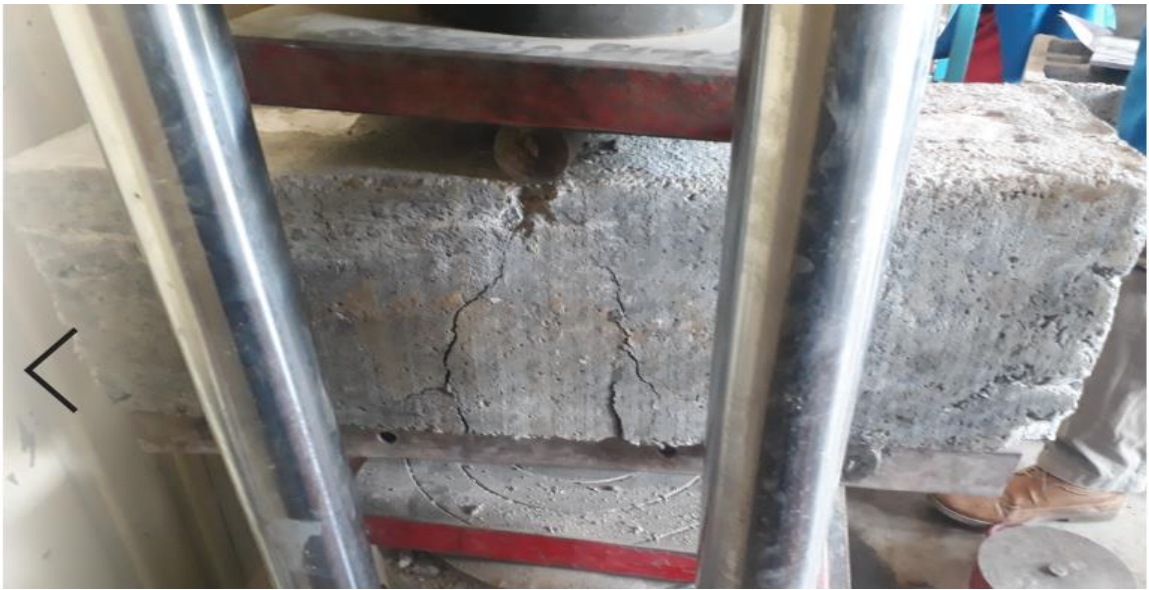
Figure 4.37. Crack of RC beam without glass fiber
