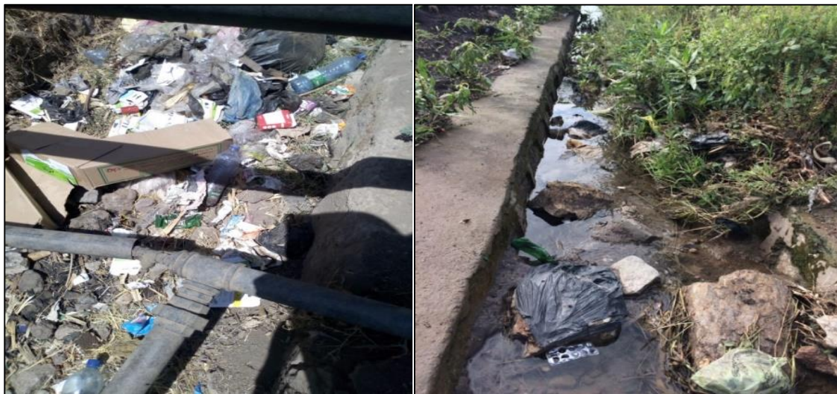
Figure 4.2: Blockage of the drainage system by waste materials
