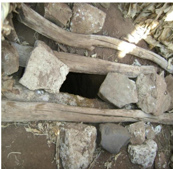
Fig.7.1 Pit latrine with no bowel taken from Howolso Kebele
