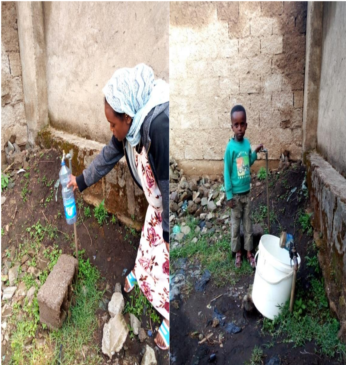
Fig 9.Old and Long Water Pipe Challenges to water distribution
