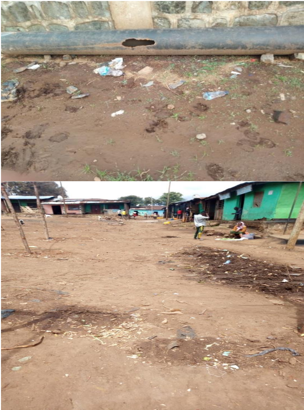
Fig 7.Unfinished water pipe stretch distribution strategies
