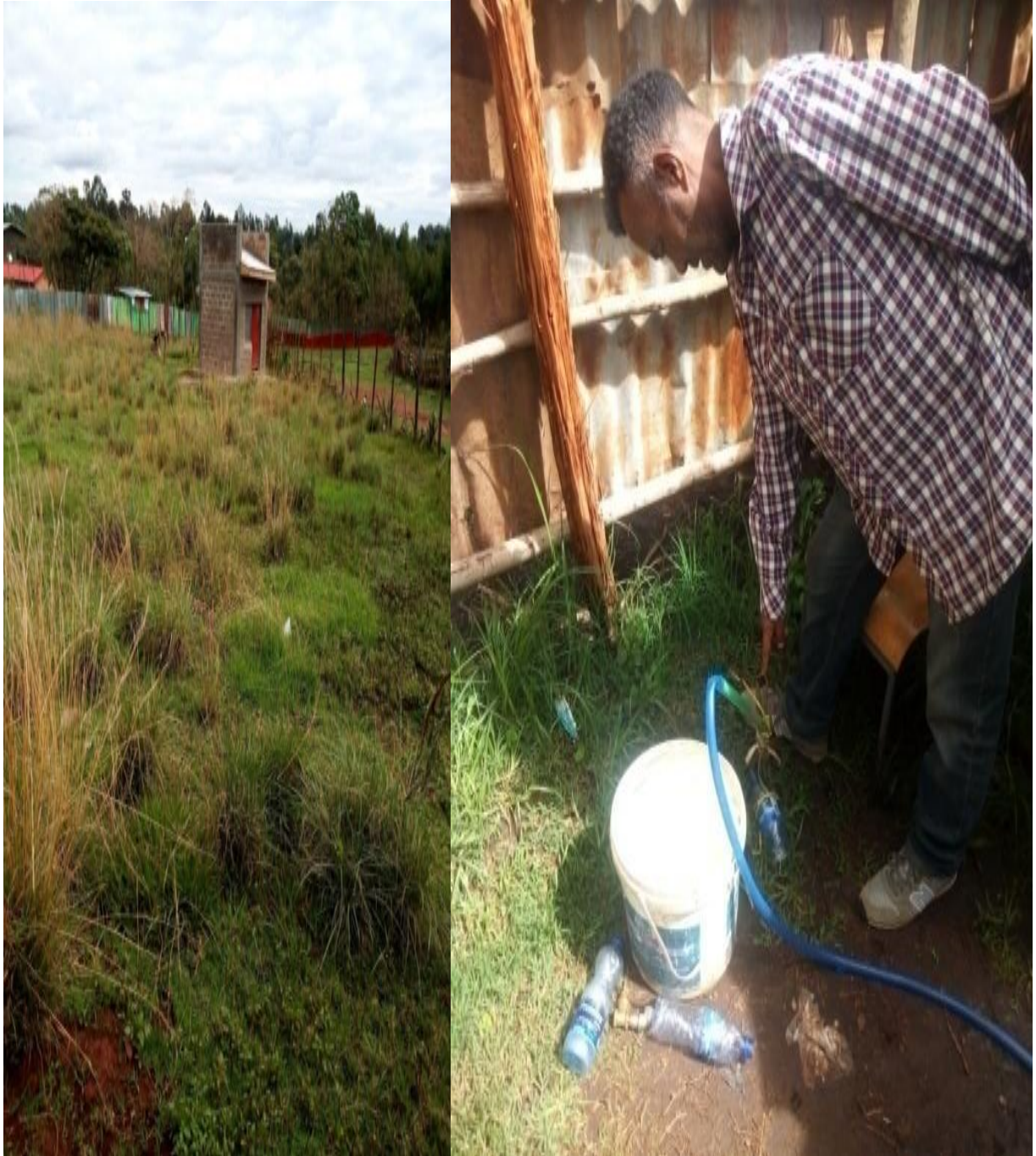
Fig. 8...Damaged water pipes and insufficient water source station
