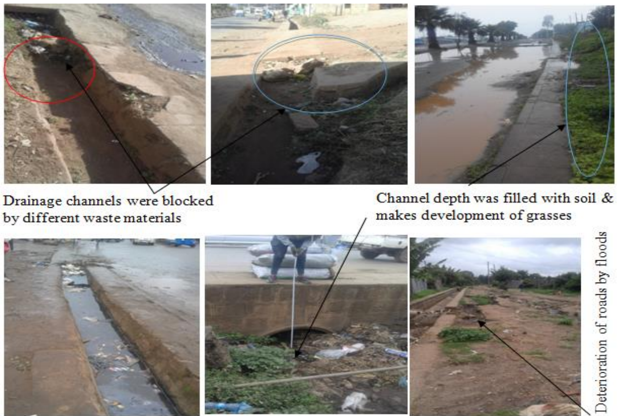
Figure 4.6: Associated drainage problems in the field (Source: field survey)
