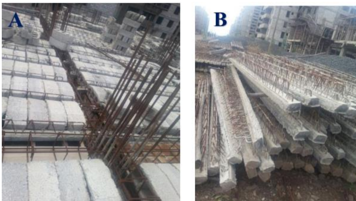
Figure 4.7 A) Ribbed slab practice in Addis Ababa condominium housing construction B) Precast beams in Addis Ababa condominium housings
