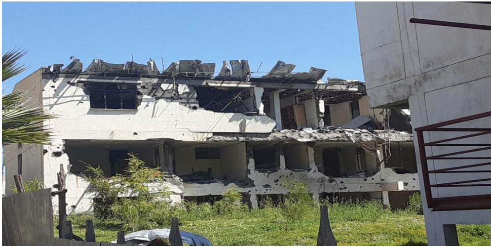
Figure 7: Damaged view of Wollo University, Main campus
