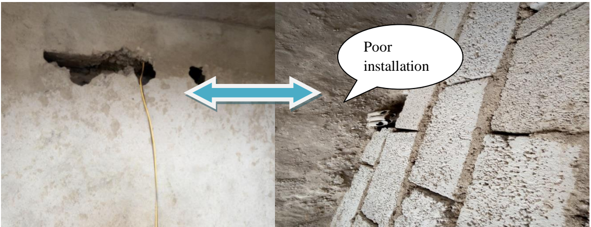
d. Poor installation and wall defects
