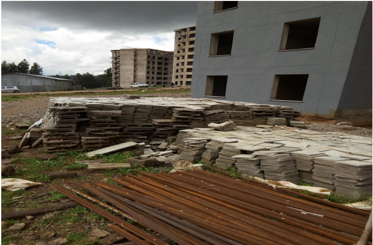
c. Hand rail making steel exposed to corrosion
