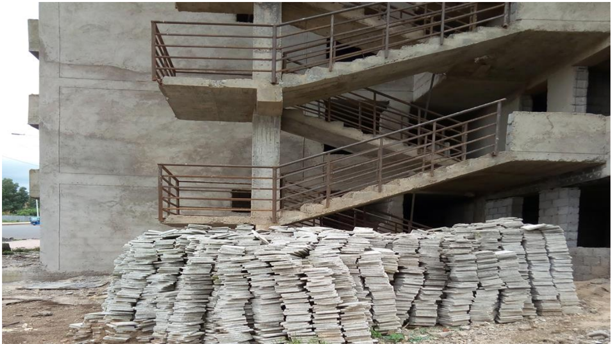
b. Terrazzo for the flooring stored wrong manner
