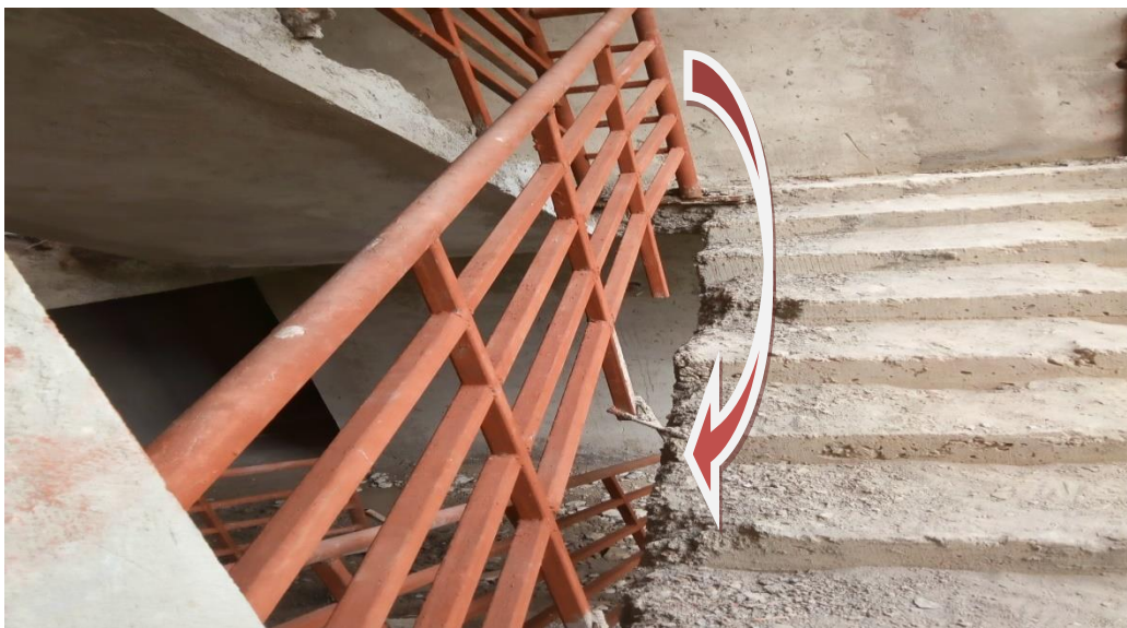
b. The handrail is fixed away from the stair
