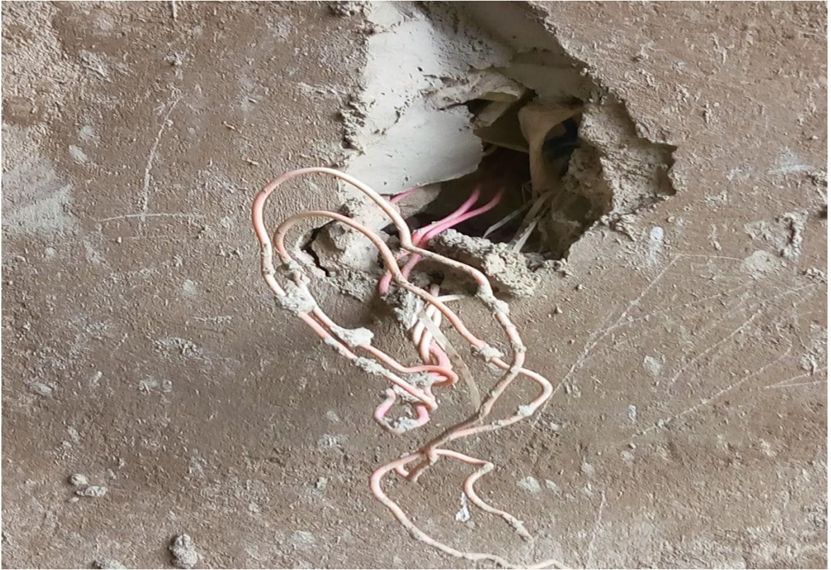
c. Defects on electrical installations and wall
