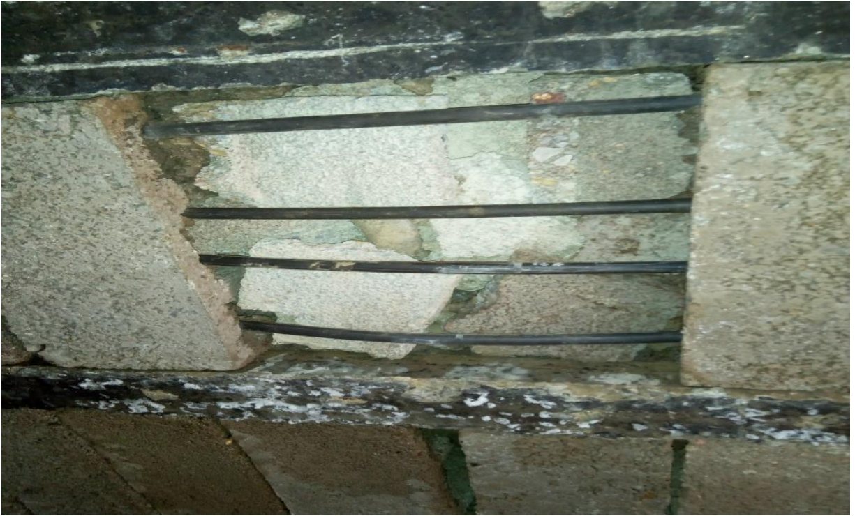
a. Electric cables line does not covered in the slab
