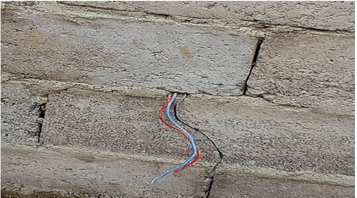
b. Electric wire is out of the conduit
