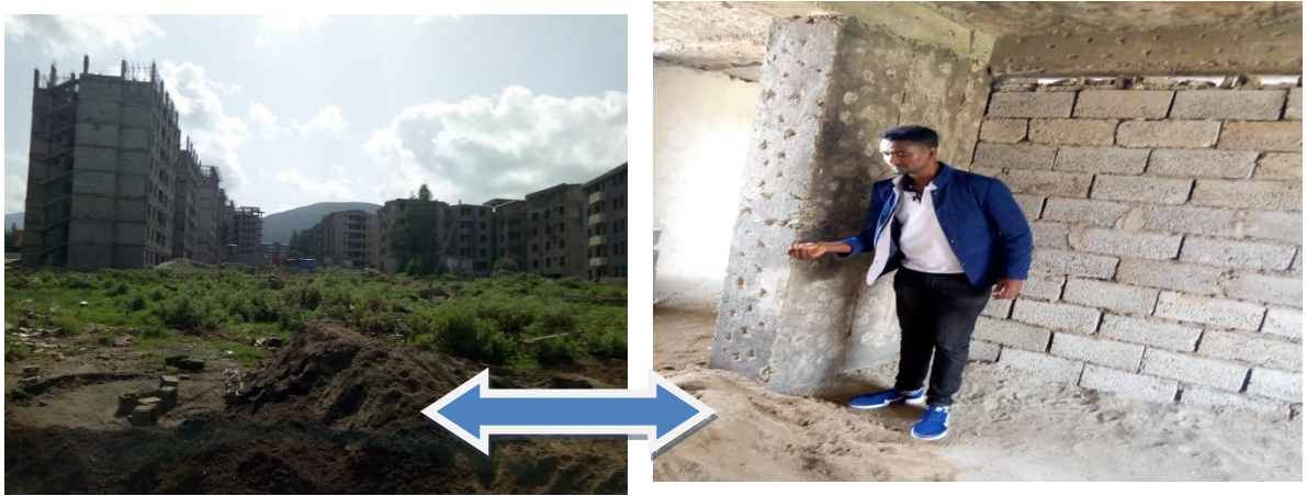
a. Low quality fine aggregate and poor handling on the site
