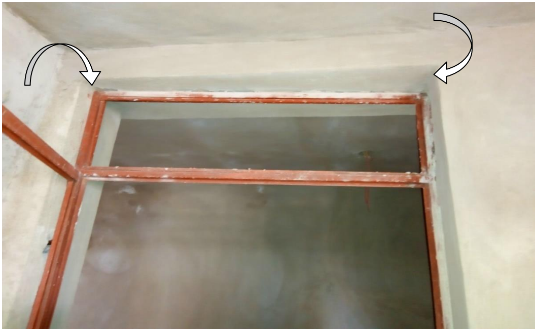
a. Defect on fixing of the door
