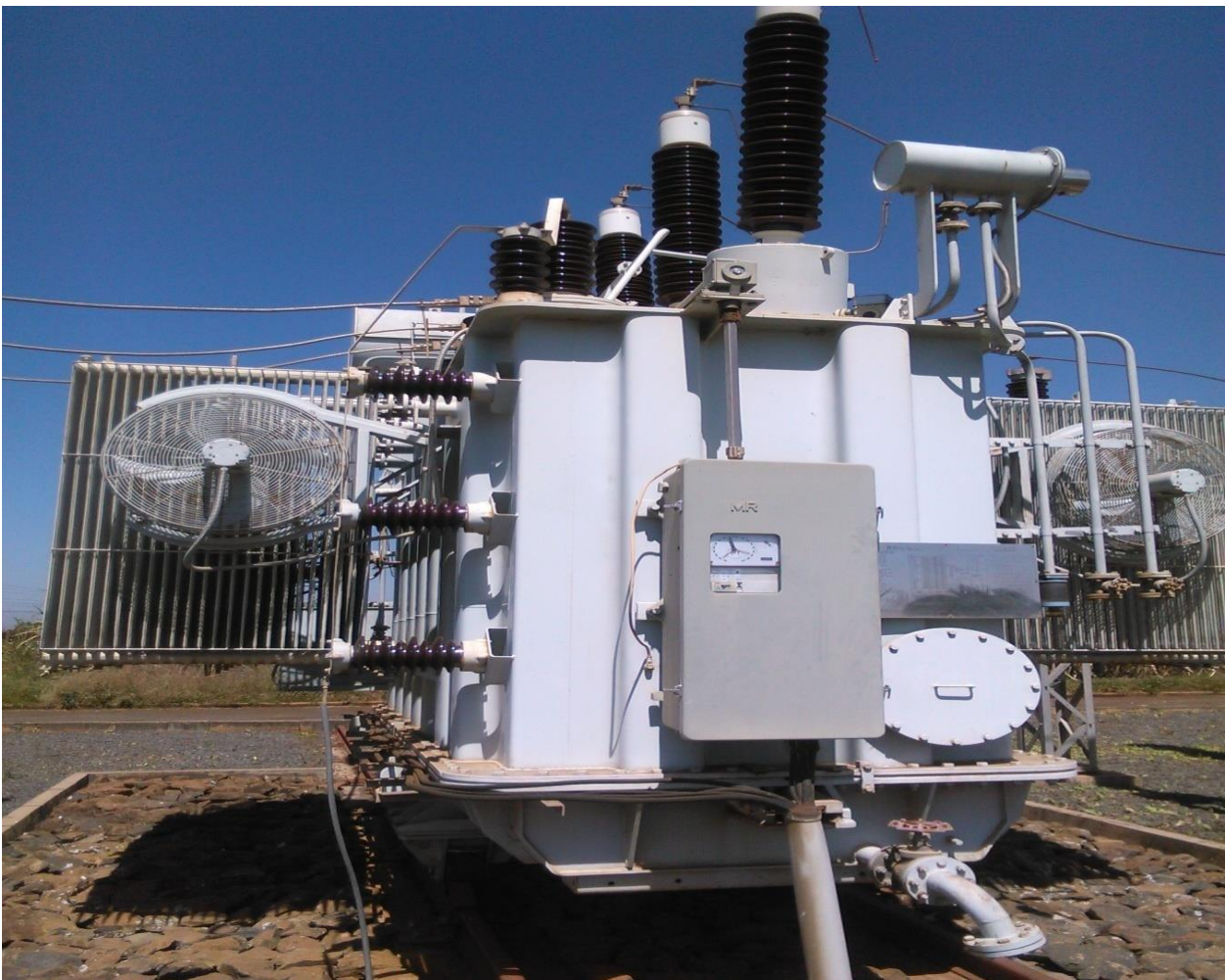
Figure 3.4: 132/15KV Power Transformer Photo in Bule hora Substation
