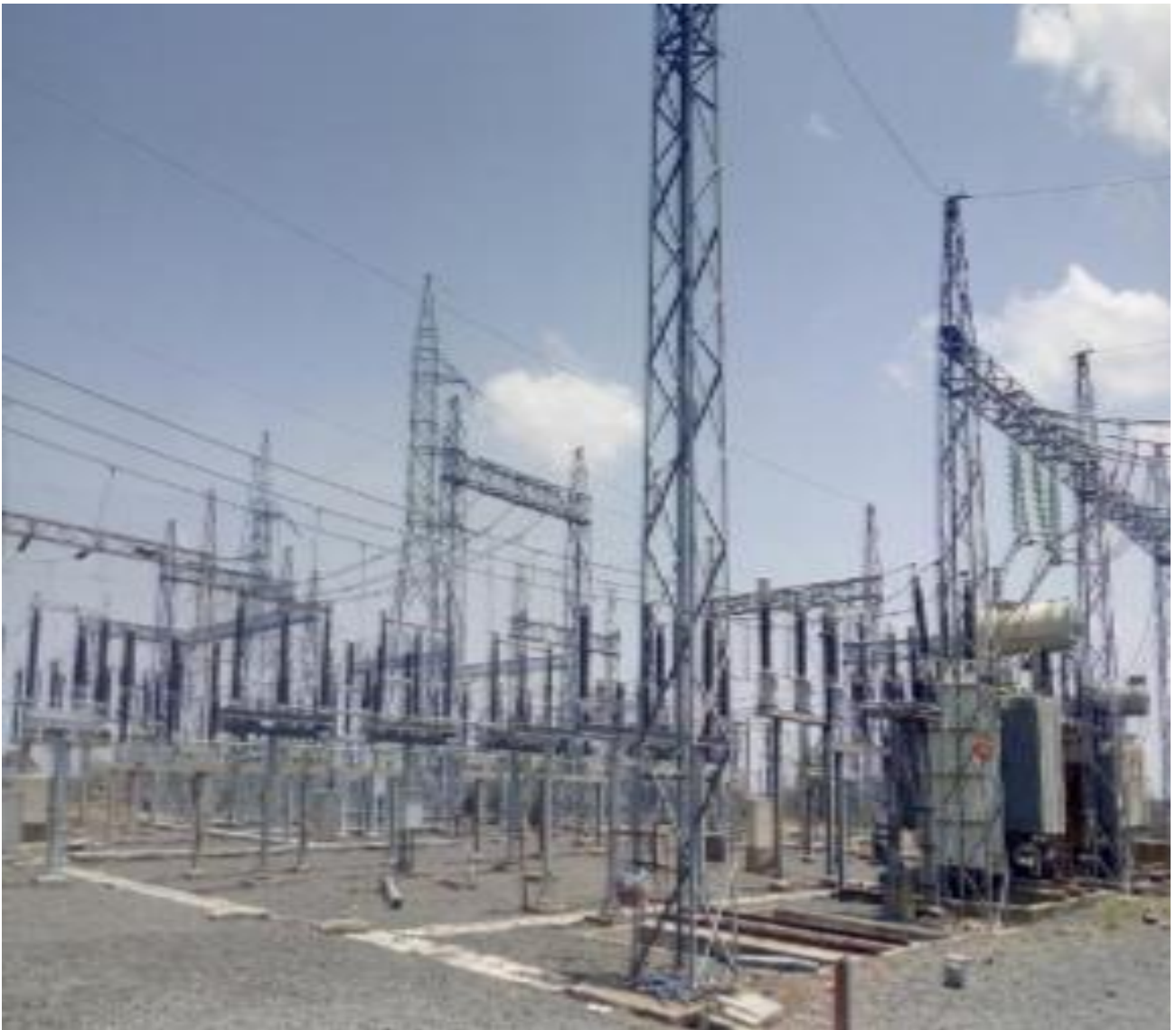
Figure 3.3 Bule hora Substation [Source: study area]
