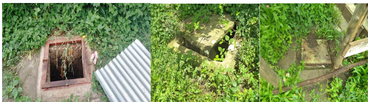
A. Basha health center B. Aruma health center C. Kella health center Figure 5: Placenta pits in a, b&c (Basha, Aruma and Kella health center respectively)
