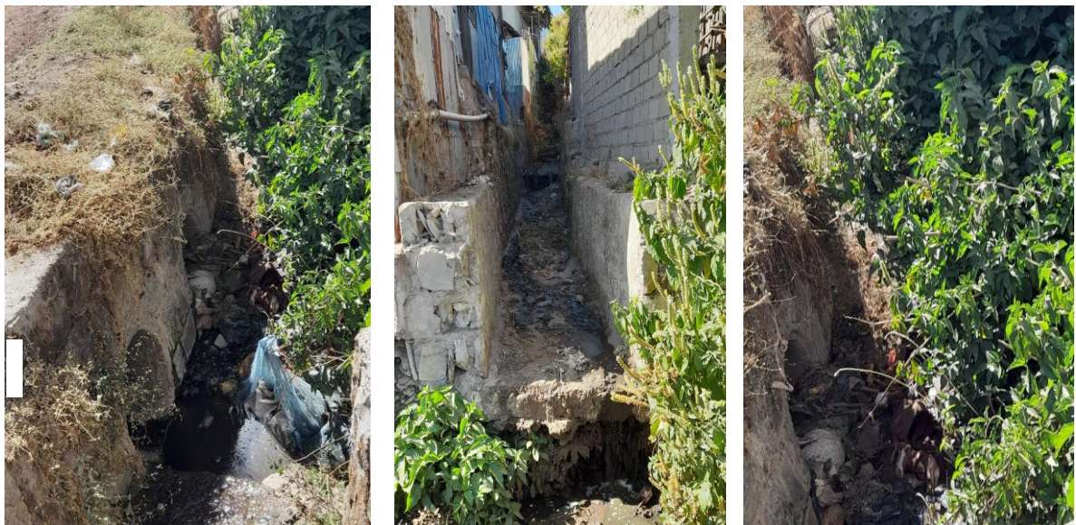
Figure 6: Damaged drainage structure due to settlement of soil and constructed drainage structure at bottom side of residential, tenatabiya sefer(site visiting time)
