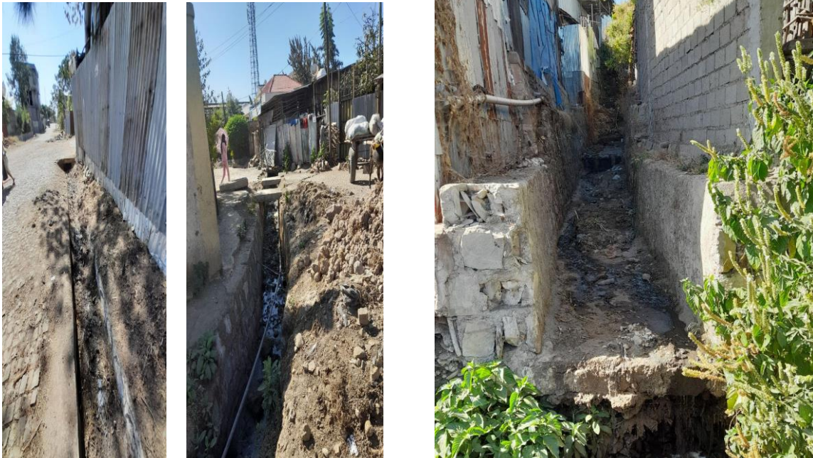
: Figure 10 :Placement ,Mis Use, poor alignment of drainage structurs(site visiting time)
