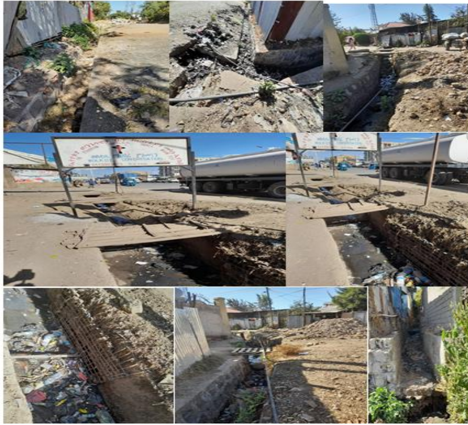
Figure 14: Sample of uncovered drainage ditches in the study area( site visiting time)
