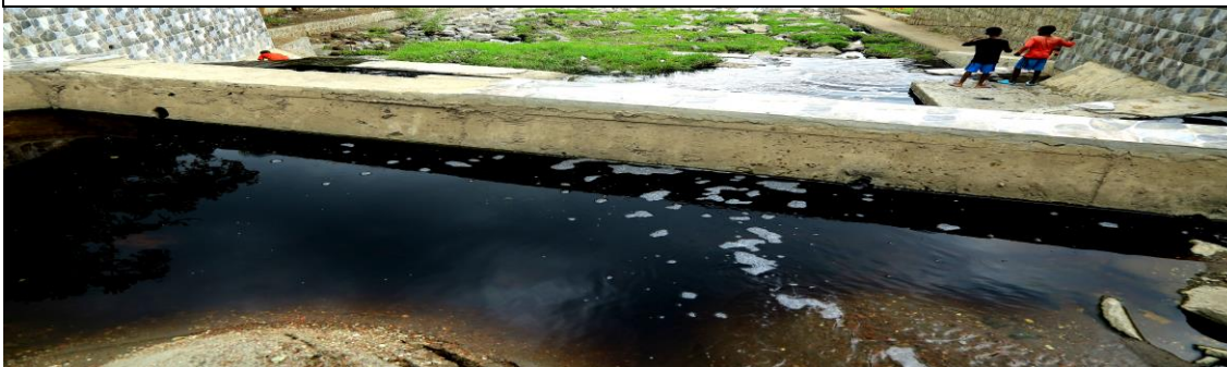
Failed storm water in Gudumale kebele
