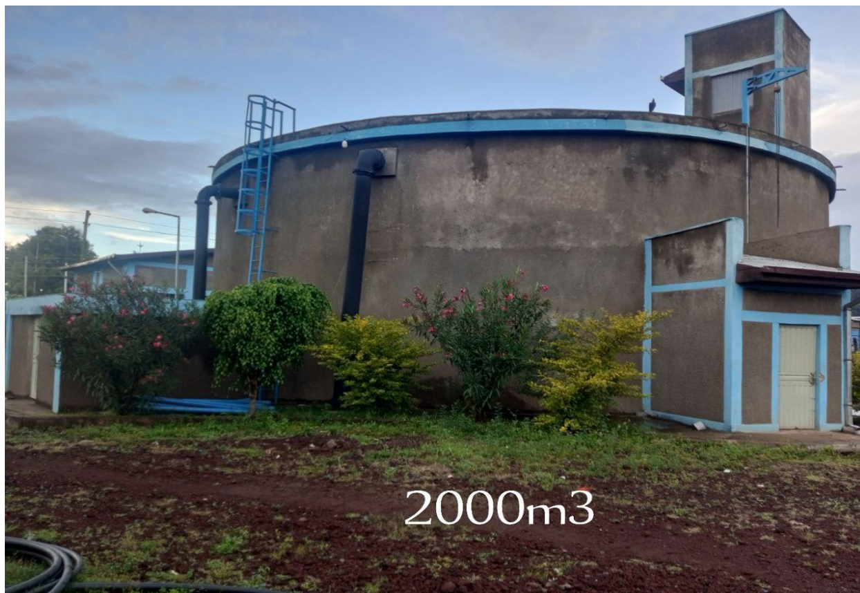
Figure 3 3: The existing 2000m3 reservoirs in the town
