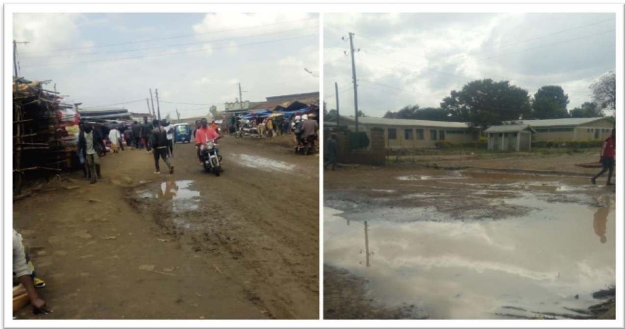
Figure 8: Deterioration of asphalt road around existing market and stagnation of water on the rightway in front of Aleta-Chuko Primary Hospital respectively
