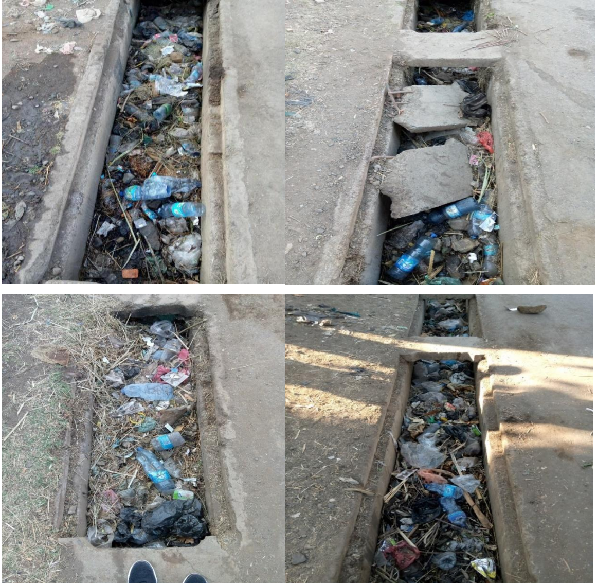
Figure 4.8: Deposition plastic materials in to drainage ditches (site visit)
