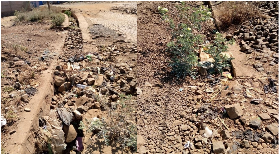
Figure 4.10: Clogged and broken outlet ditches
