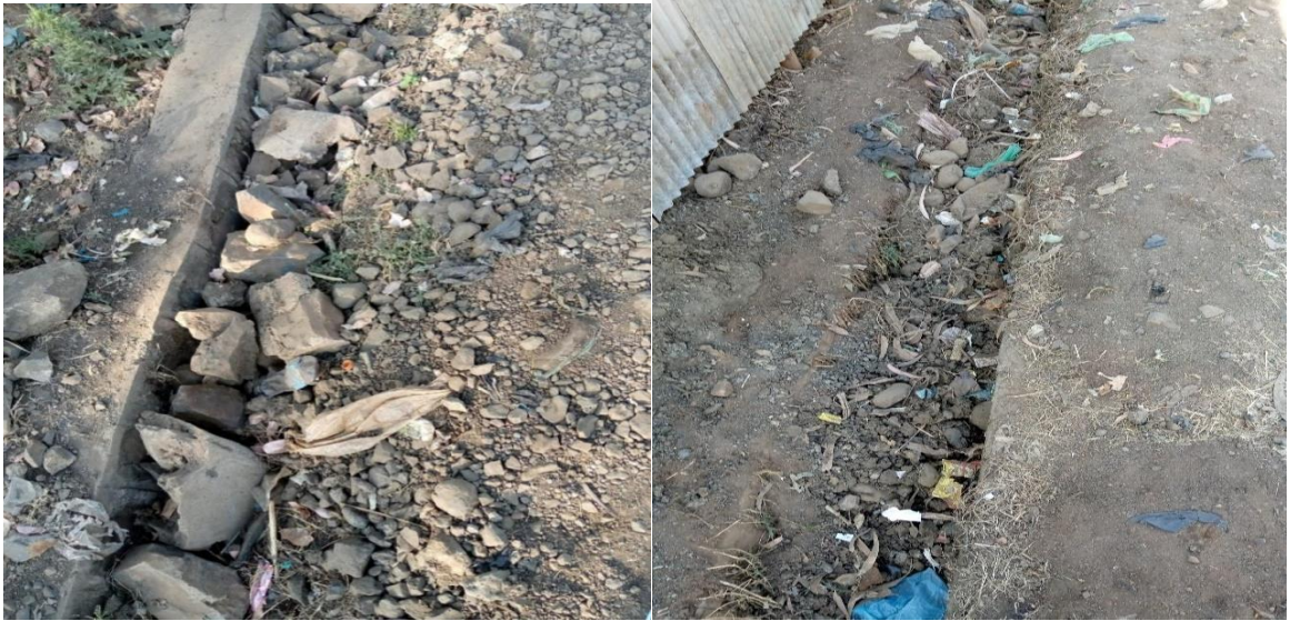
Figure 4.9: Broken road side ditches (site visit)
