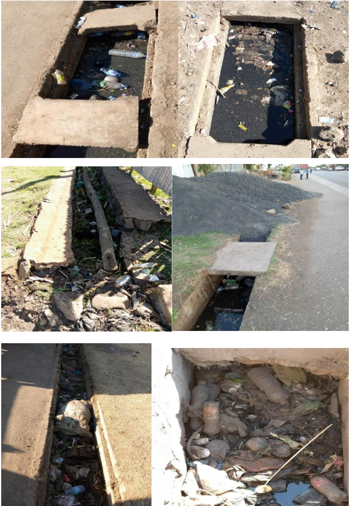
Figure 4.7: Clogged structures with electric poles, construction materials, and disposed wastes (site visit)
