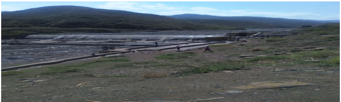
Figure 3: Golina irrigation headwork structure
