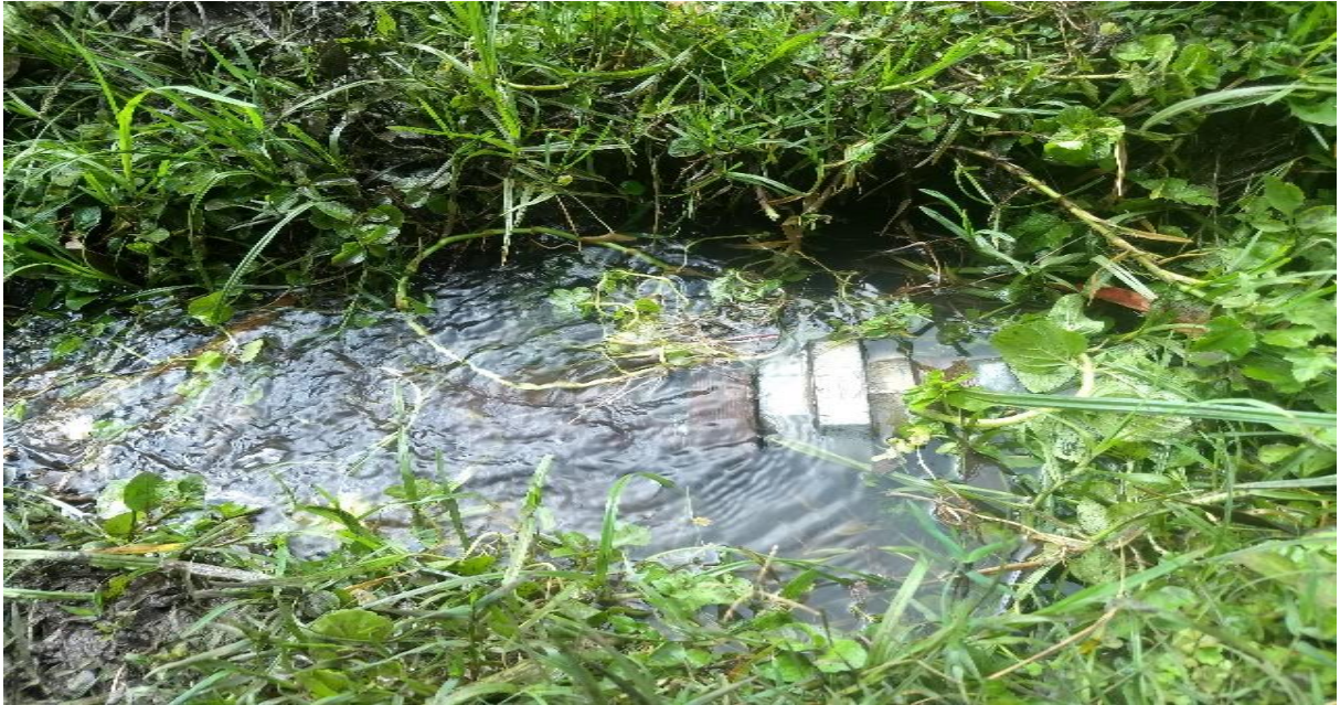
Figure 3.5: Existing water loss by leakages
