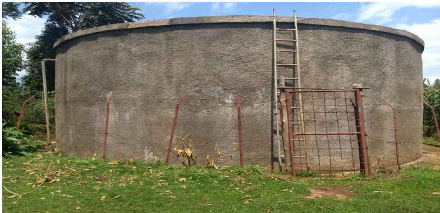
Figure 3.2: Service Reservoir 500m 3
