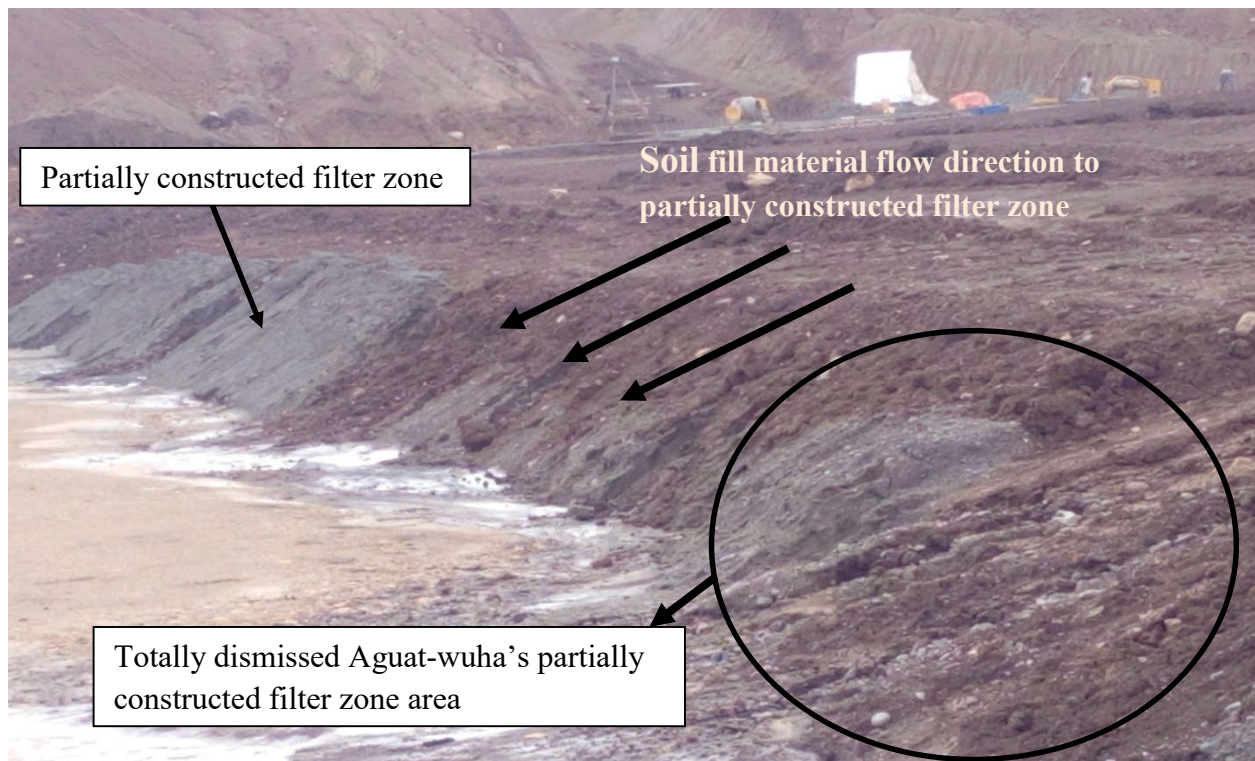
Figure 9: contamination of partially constructed filter zone
