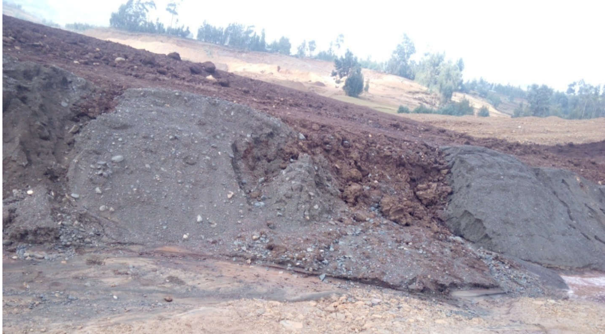
Figure 10: contaminated by fill soil and loose serviceable partially constructed filter zone
