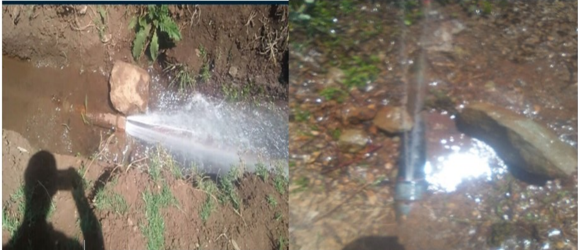
Figure. 4.4. Picture of leakage due to poor Maintenance
