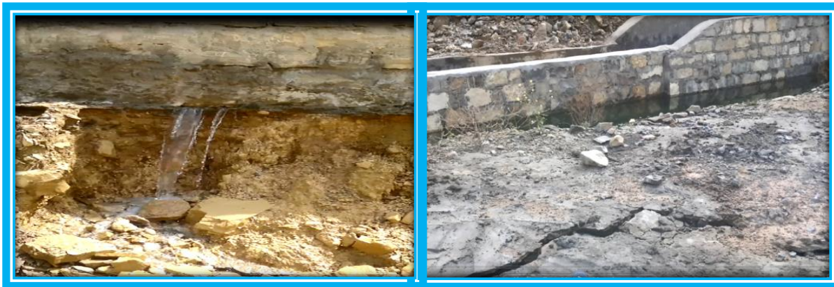
Figure 4 5: situation foundation of the spillway and the canal around the out let
