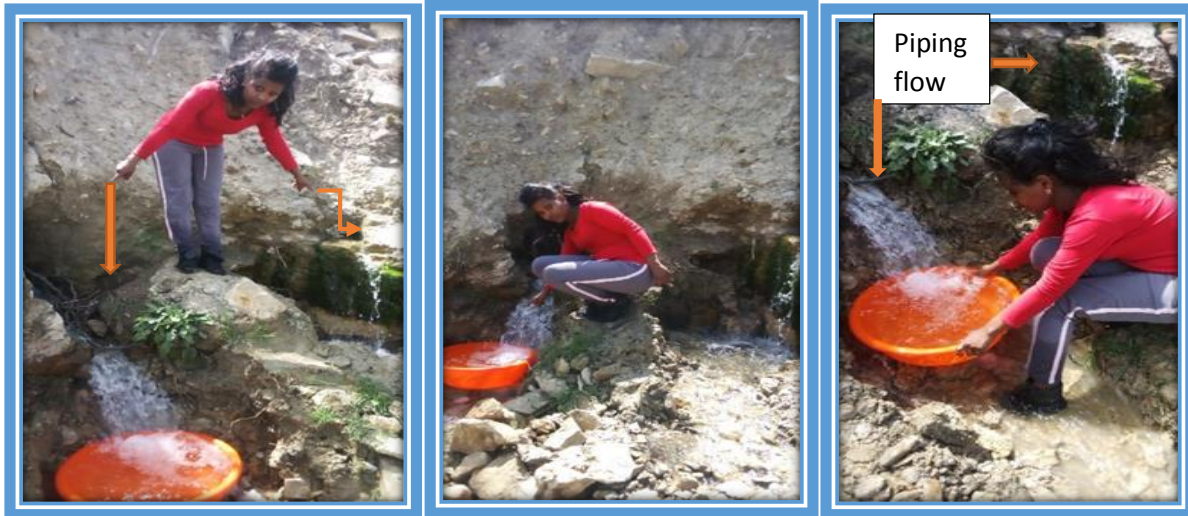
Figure 3.6: current seepage measured on Grindeho dam at the left abutment (February, 2017)
