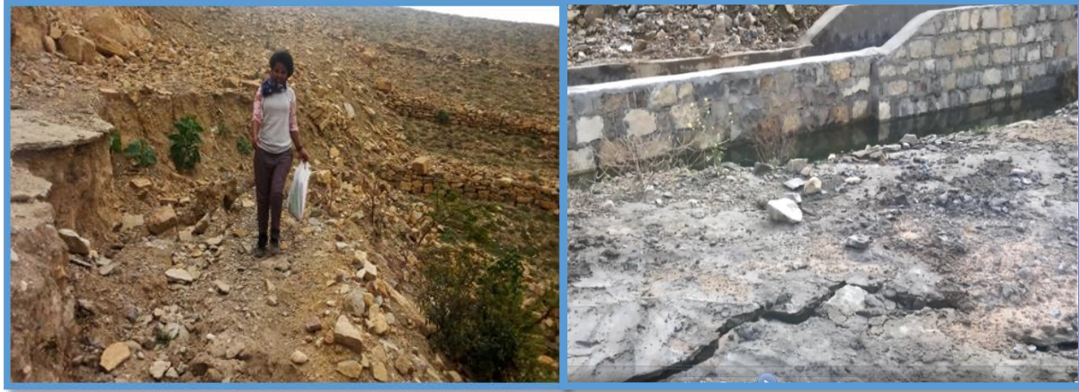
Figure 4.4: Land slide situation near the spillway and the out let
