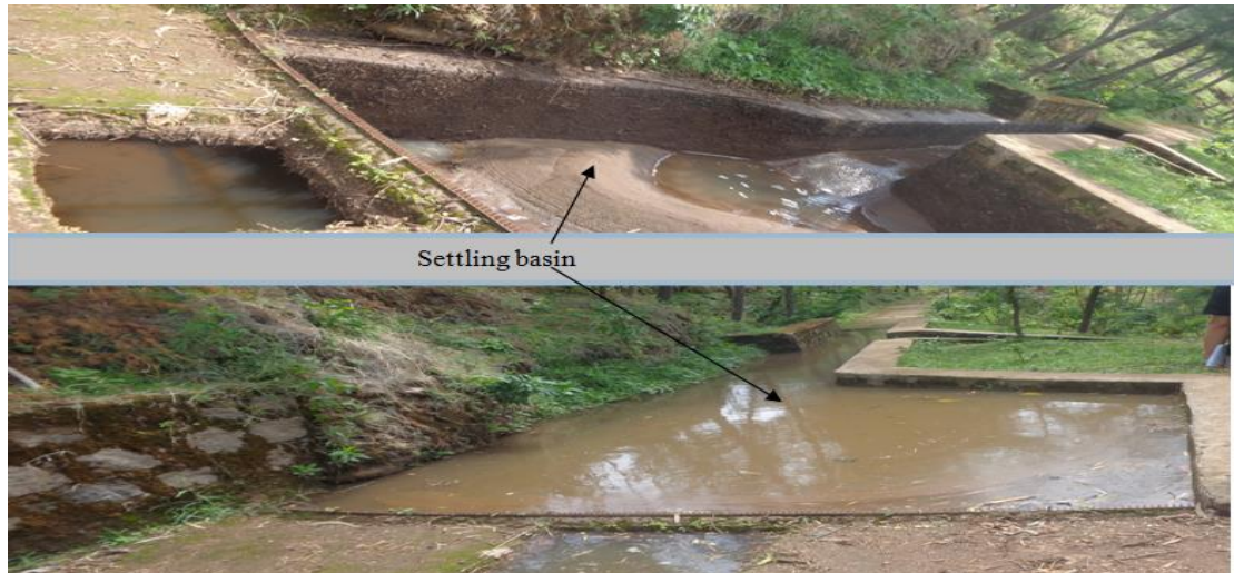
Figure 4-10:- Sedimentation problem of at settling basin of Lelta MHP
