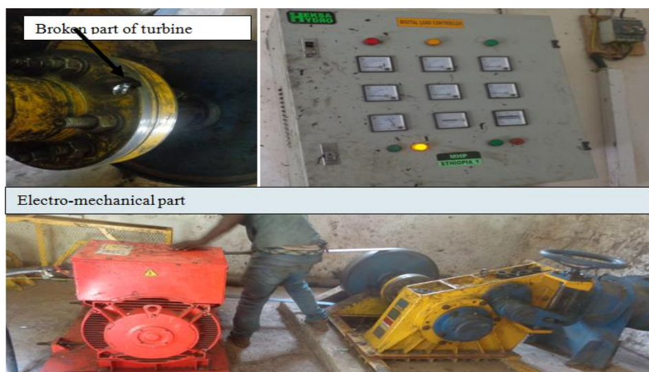
Figure 4-9:- Electro-mechanical part of Lelta MHP
