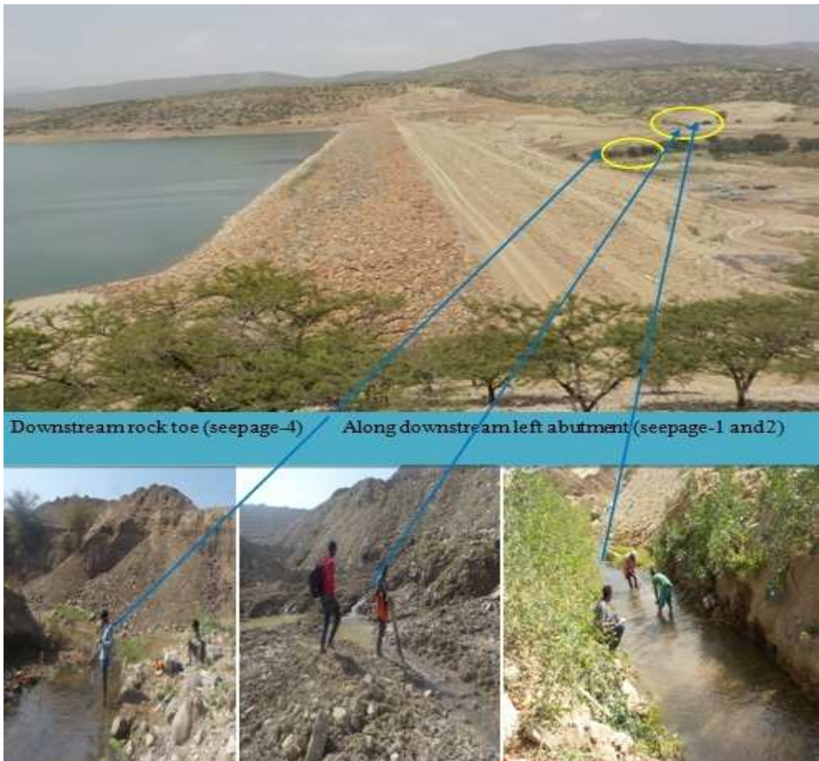
Appendix Figure E: location of seepage on the downstream area of the dam.
