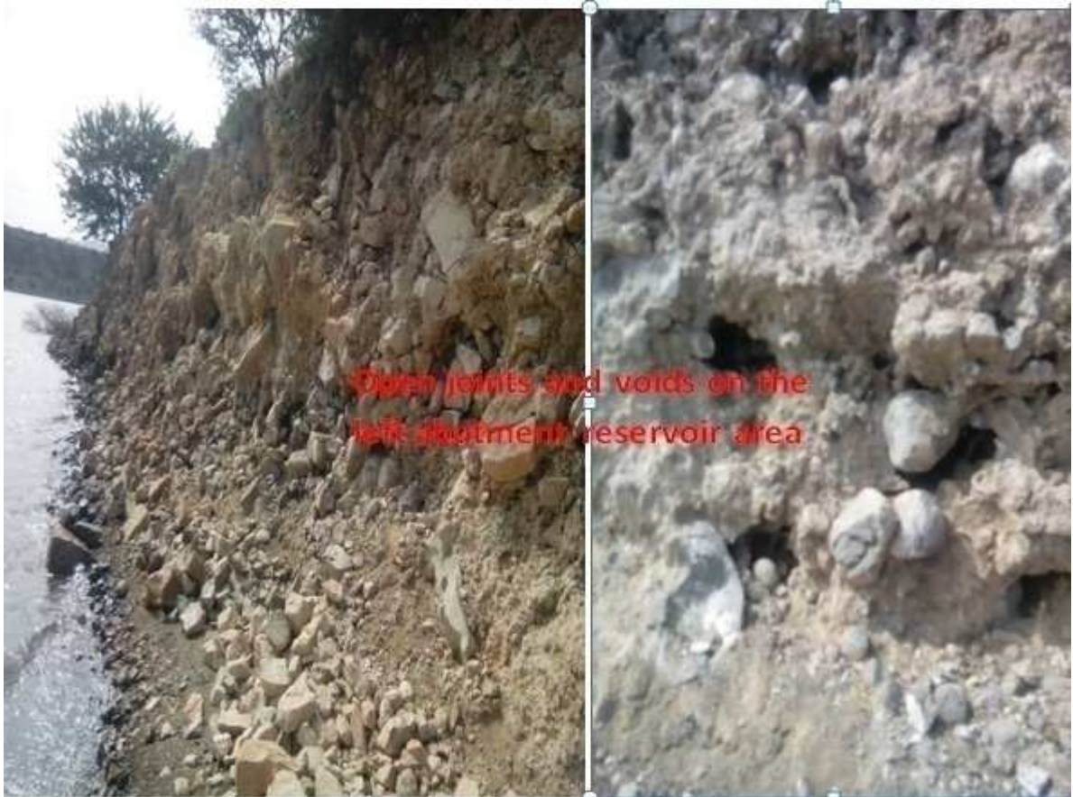
Appendix Figure G: Photographs showing the weathering open jointed and voids on the left reservoir rim area.
