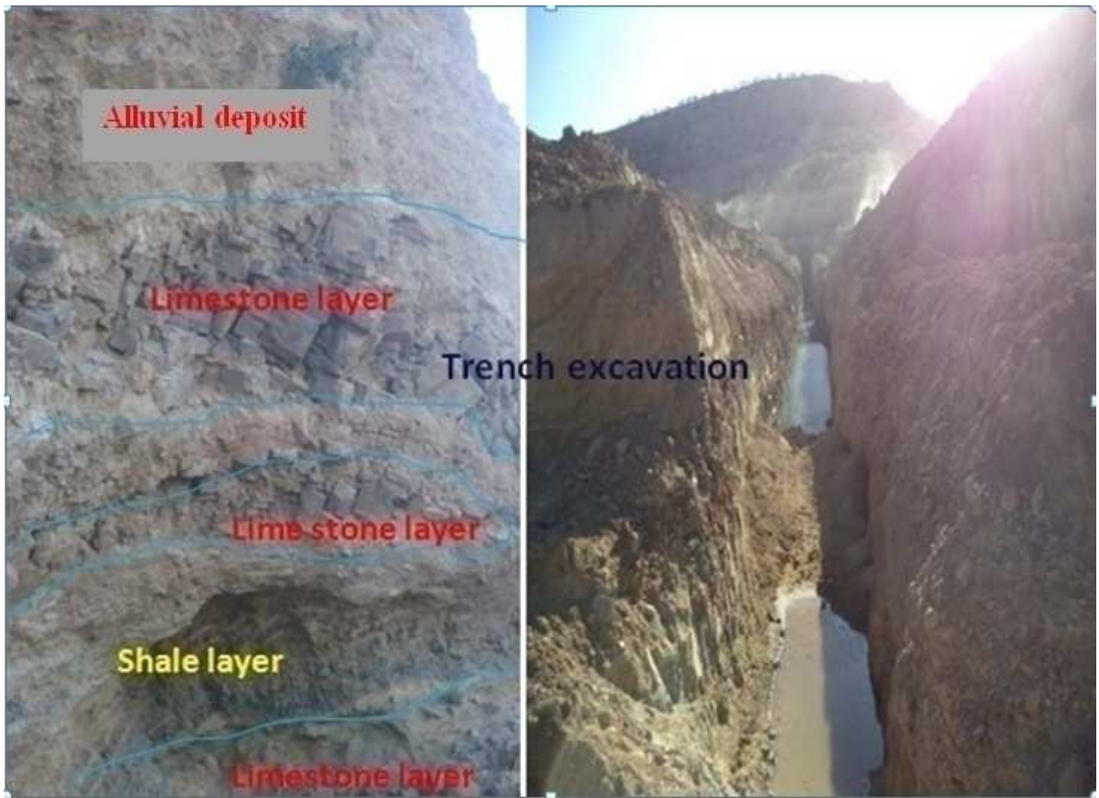
Appendix Figure F: during the trench excavation of the geological foundation (shale-limestone intercalation in the Gerebsegen dam).
