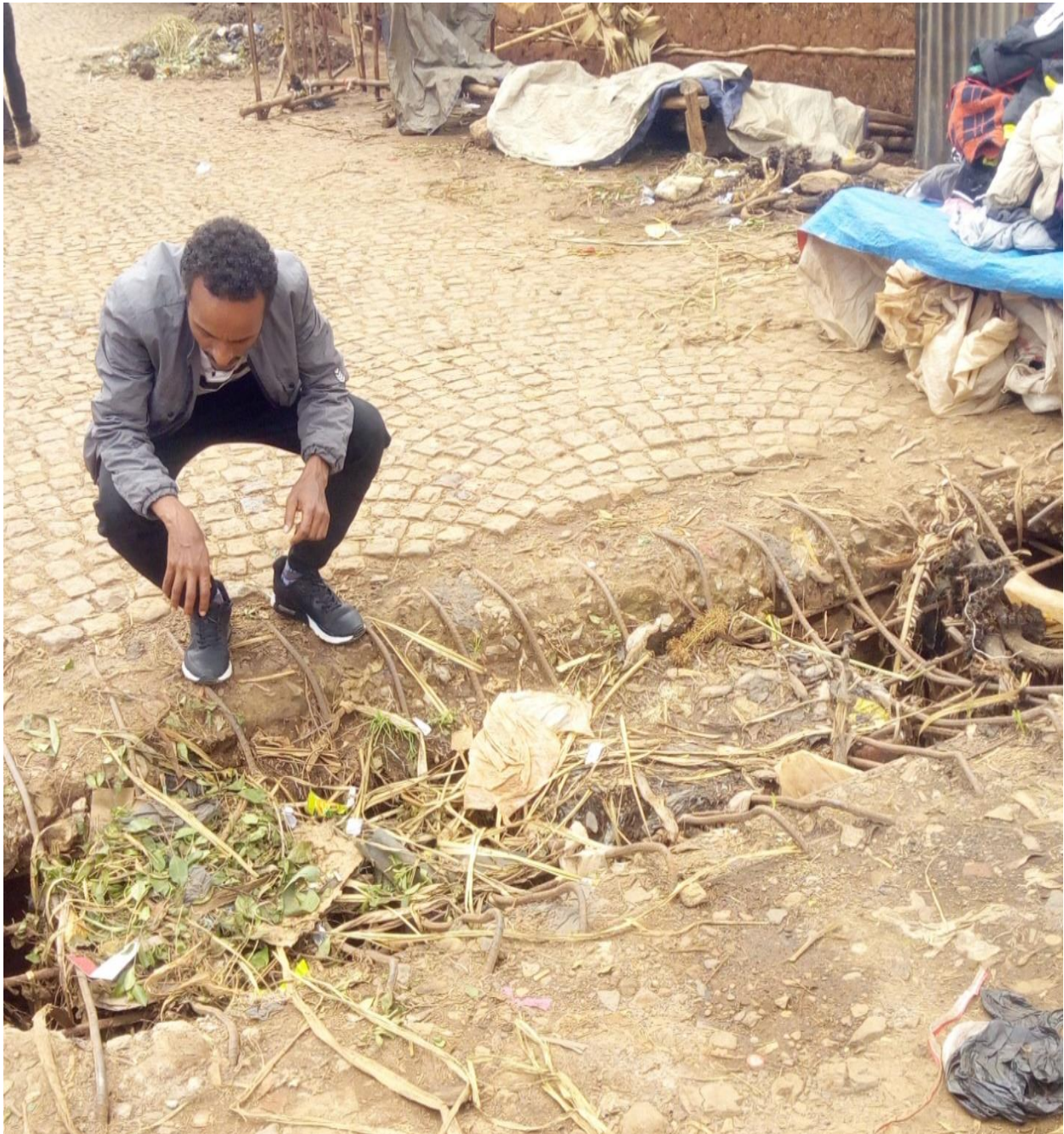
Figure 4.5 Failed drainage system by the dumping of solid waste
