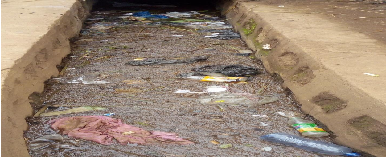
Figure 4. 17 shows blocked ditches in the study area
