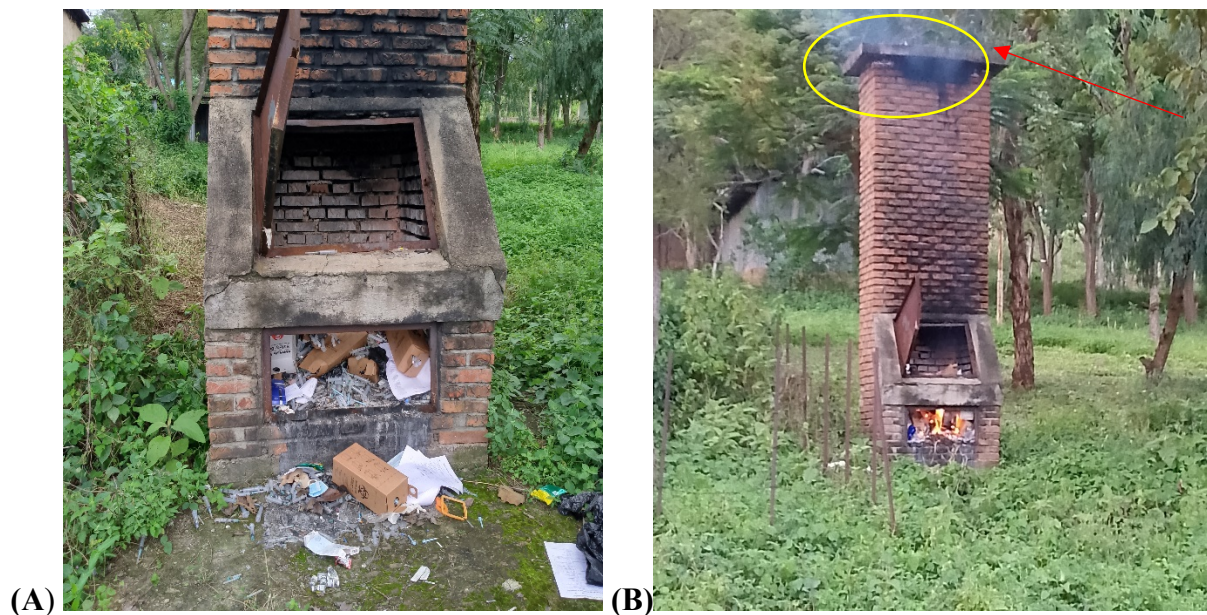
Figure 11: Photo shows the incinerator site (figure A), firing the waste loaded to the incinerator and smoke emission (figure B), in Kelle Primary Hospital, February 2024
