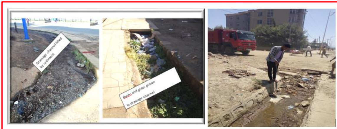
Figure 19: Drainage Facility Filled by Sediment and Solid Waste
