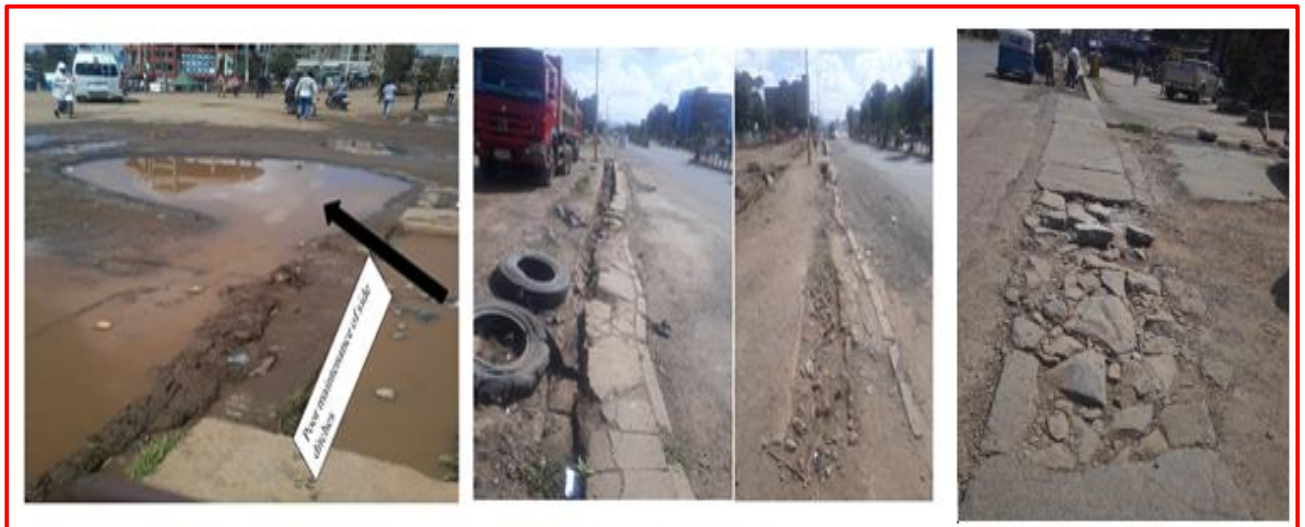
Figure 18: Ponding of Storm Water on Asphalt Road and deteriorated road side ditches. (Field survey, 2011).
