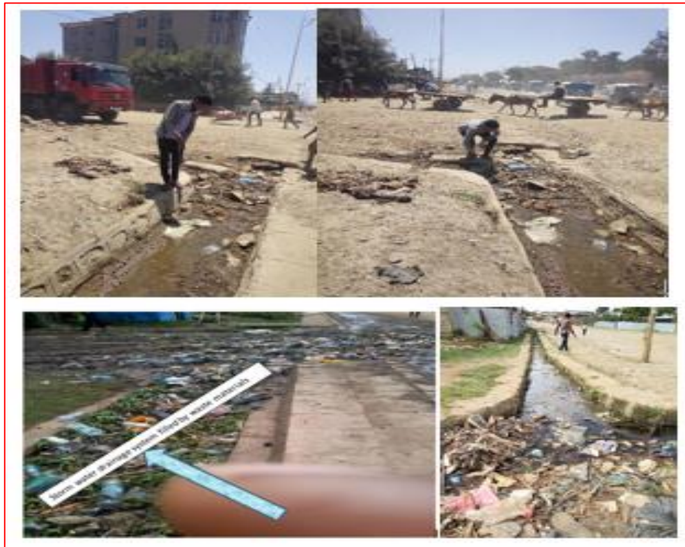
Figure 6: Field survey and problem associated drainage System
