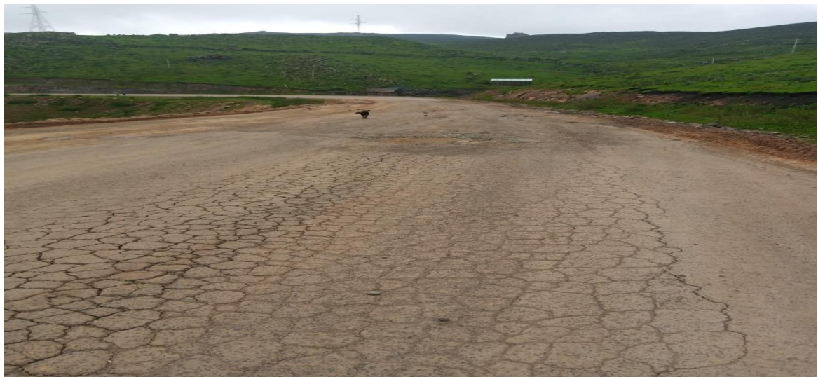
Figure 4-1 Alligator cracking and rutting failures observed at location around 375+000km
