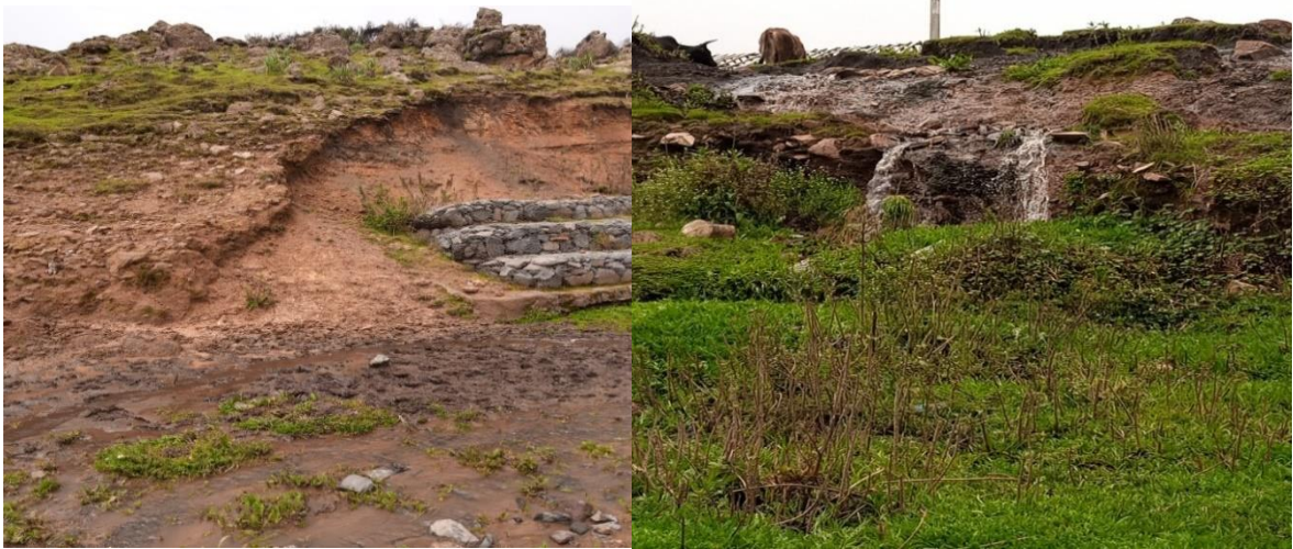
Figure 4-3 Geological profile the road and falling flow of ground water from upper hill at location around 377+000 and 376+000
