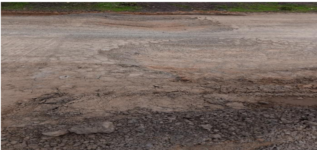
Figure 4-6 Sudden progresses of alligator cracking and potholes at transition of flexible pavement and rigid concrete slab 375+800km
