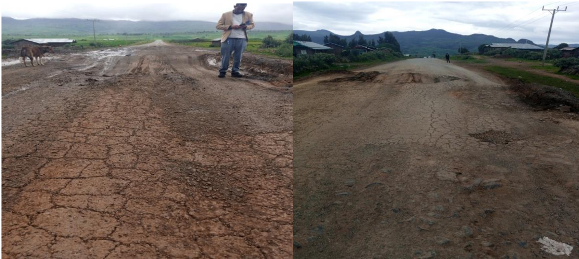
Figure 4-7 Alligator cracking, potholes and rutting type road failure at station 386+800 and station 388+300.
