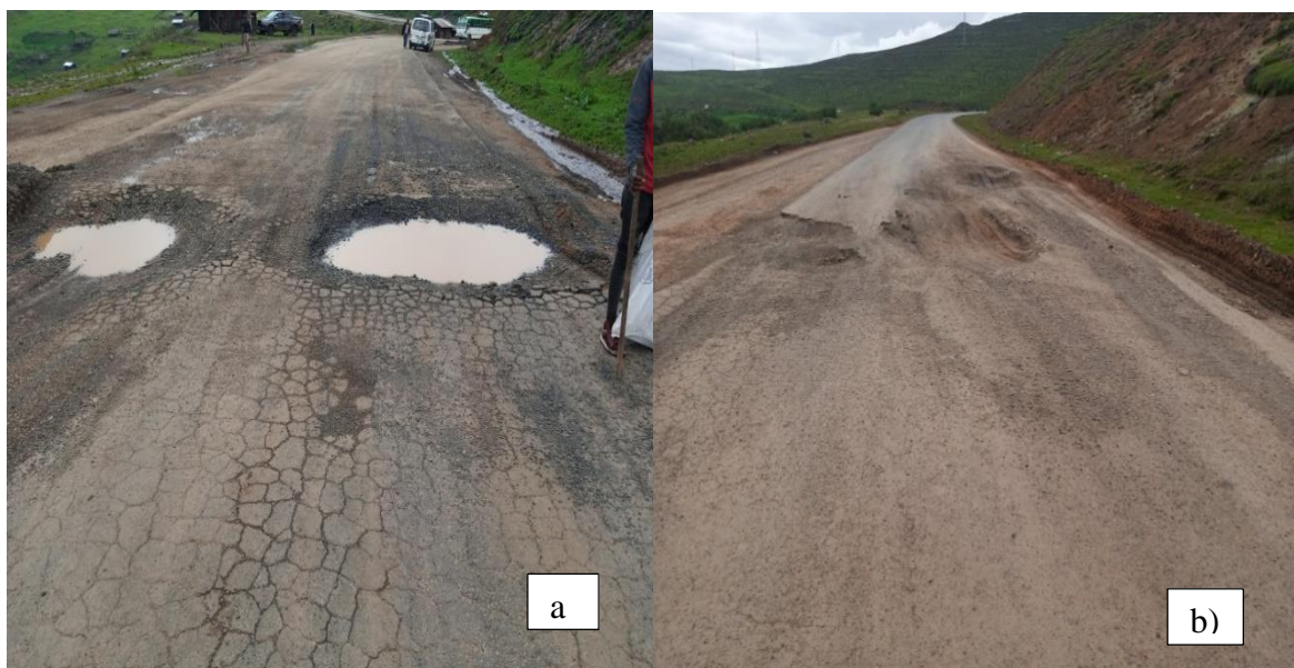
Figure 4-2 a) Water ponds on potholes failures observed at location around 377+600km.
