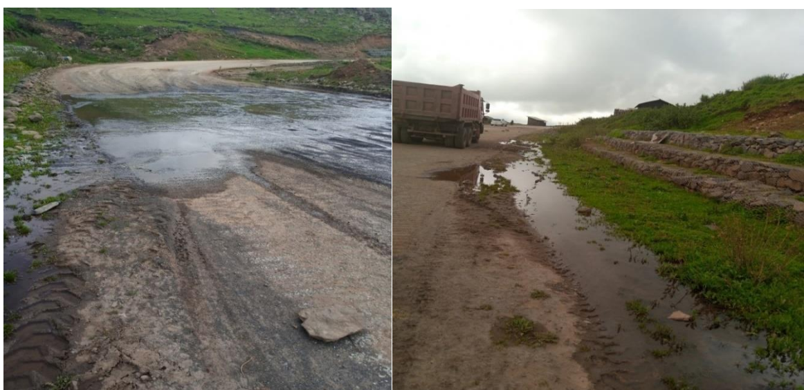
Figure 4-4 Side ditches silts up by eroded or slide soil material from hill cut slope and water falls on the surface of asphalt and shoulder location around 377+000 and 376+000
