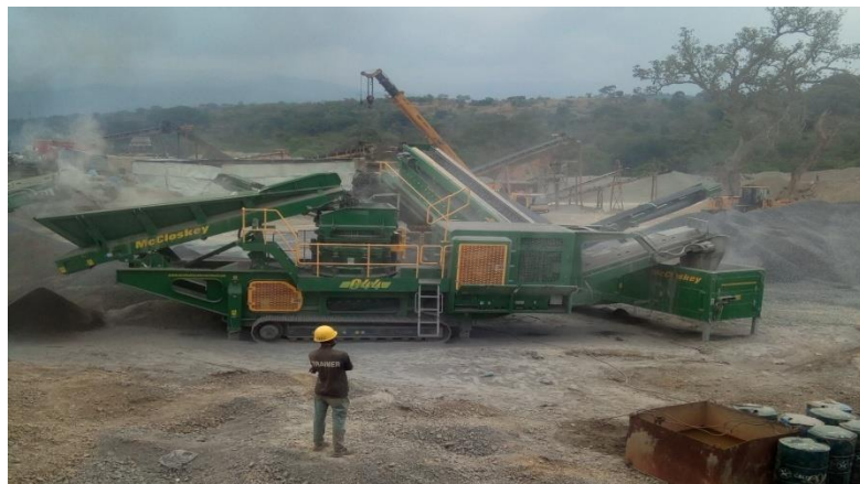
Figure 4.3 the secondary crusher (C-44) on wenago crushing site
