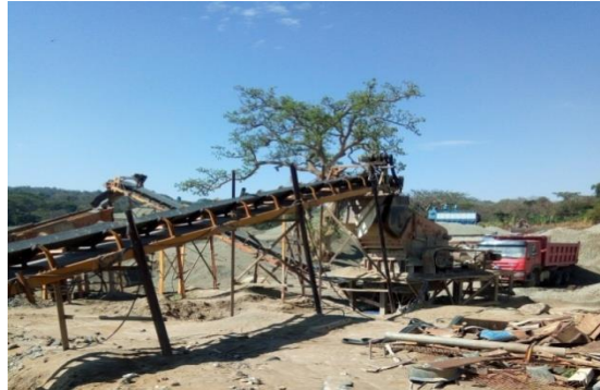
Figure 4.22 Secondary crusher of Golla crushing site
