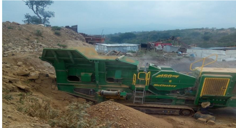
Figure 4.2 the primary crusher (J-50) on wenago crushing site
