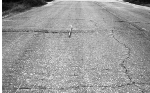
Figure2. 4 Swelling- upward displacement of a pavement
