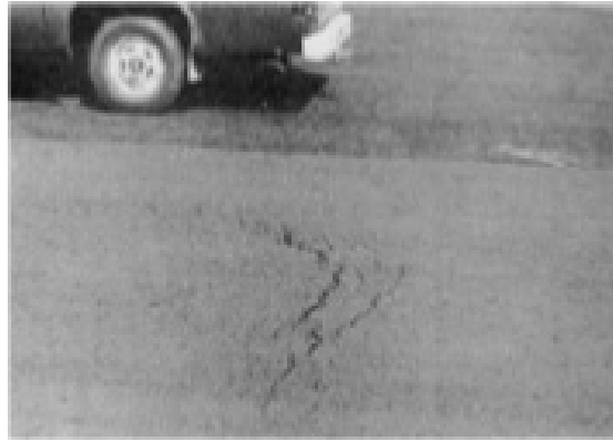
Figure2. 5 Slippage cracks (Uge, 2017)
