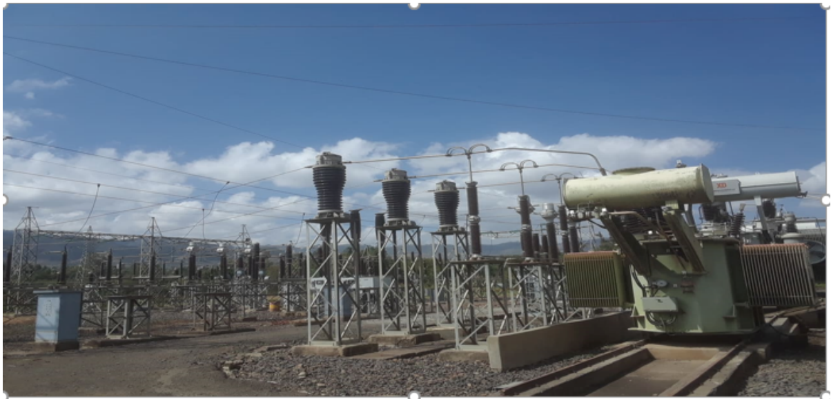
Figure 4.1: Existing substation of Kombolcha distribution network.
