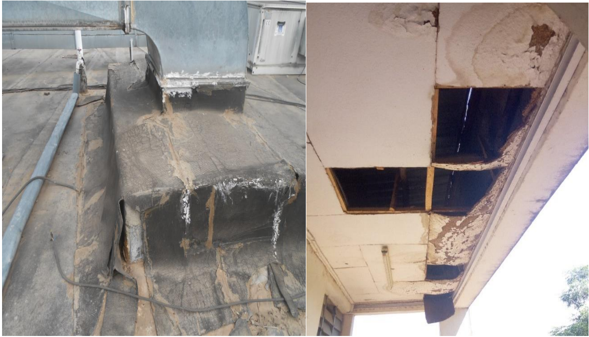
Figure 4.12 Damaged water proofing membrane Figure 4.13 Leakage effect underside roof in Dilla building (pictures taken by researcher).
