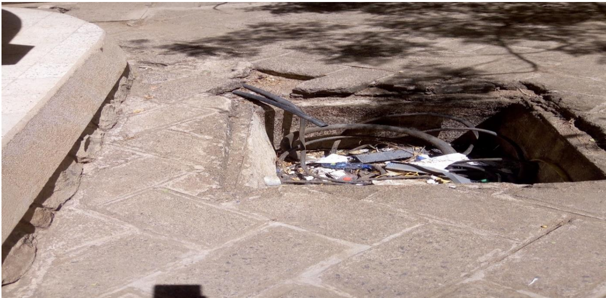
Figure D1.5. Uncovered manhole in Arba Minch University school building.(Image taken by researcher).
