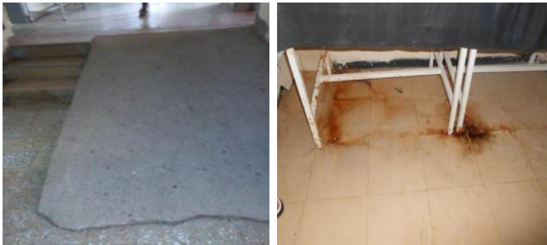
Figure 4.6 damaged ramp Figure4.7 Corroded PVC tile in hospital (image by researcher)
