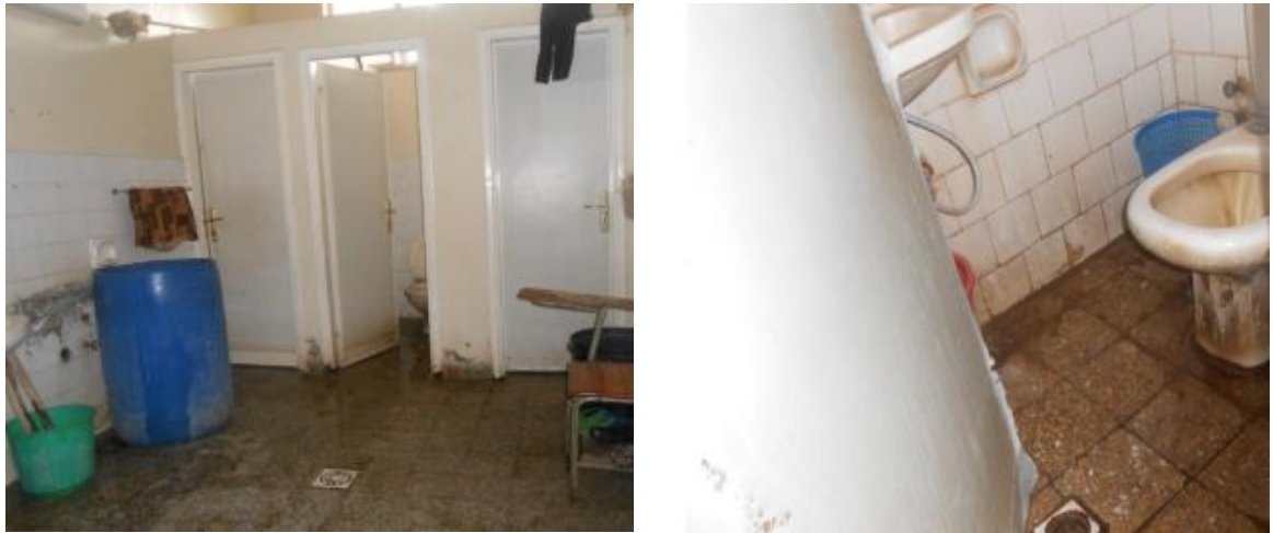
Figure 4.5 Damaged ceramic wall cladding and terrazzo tile in Hawassa referral hospital (image taken by the researcher).
