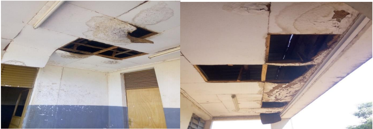
Figure D1.9. Roof deterioration on Dilla University Administration building due to EGA leakage (Image taken by researcher).
