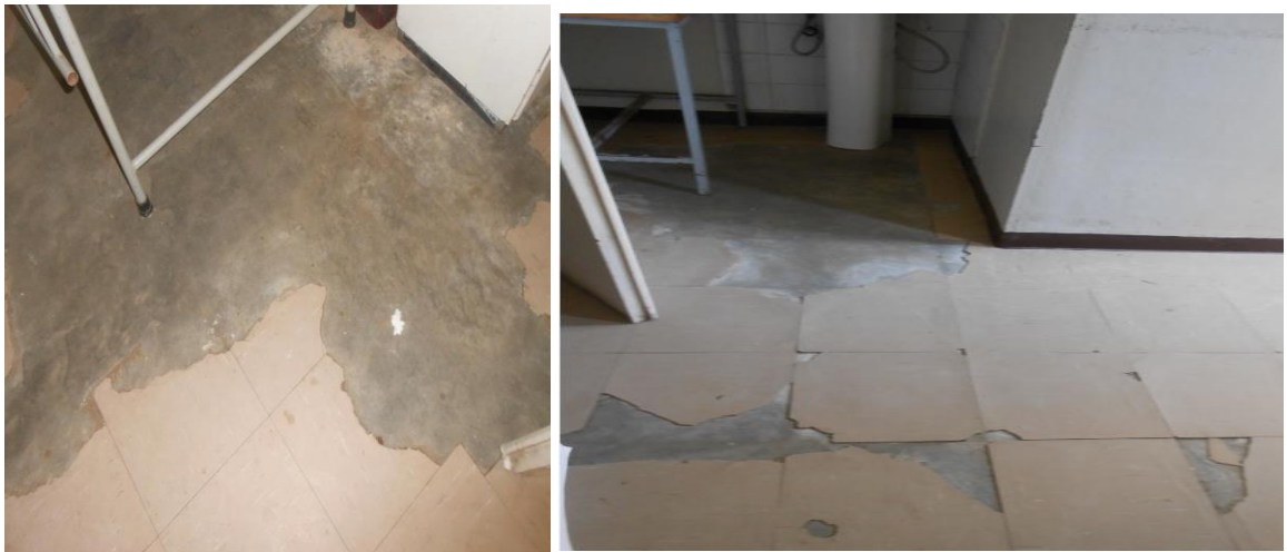
Figure 4.9 Damaged PVC floor finish at wards inpatient blocks in Dilla hospital building (Image taken by researcher).
