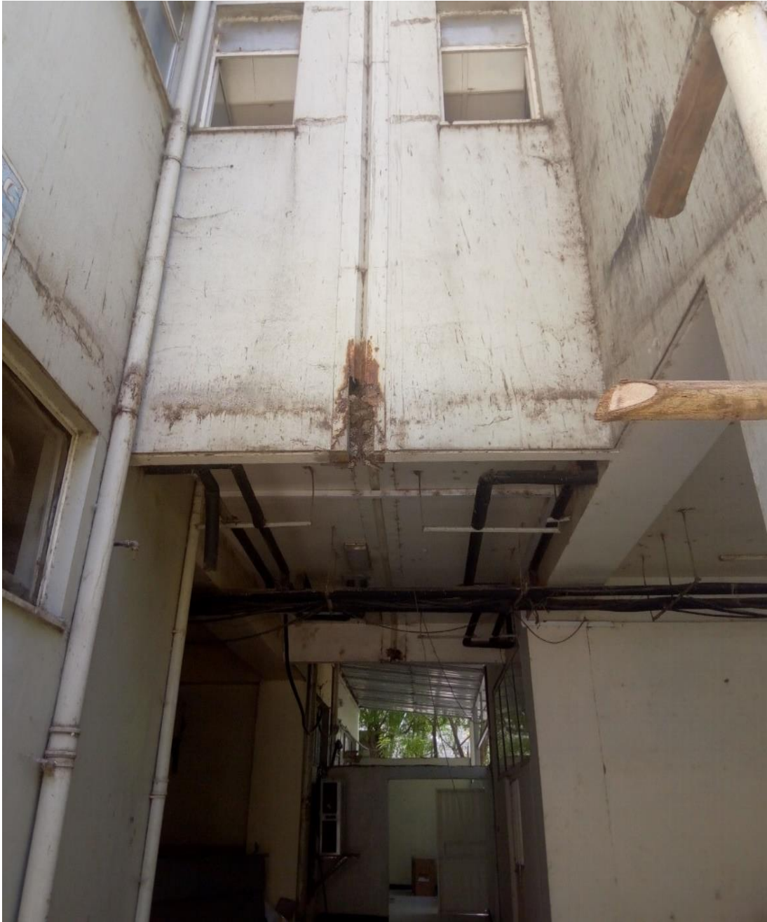
Figure D1.13. Staining and mold around expansion joint of building (Image taken by researcher).
