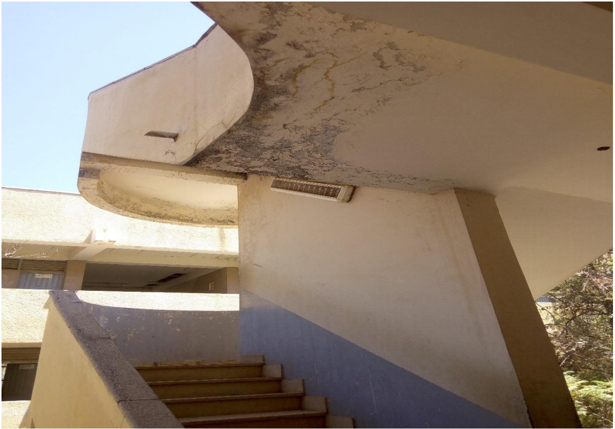
Figure.D1.6 Spalling off concrete and dampness observed under staircase of building in Arba Minch (..Image taken by researcher).
