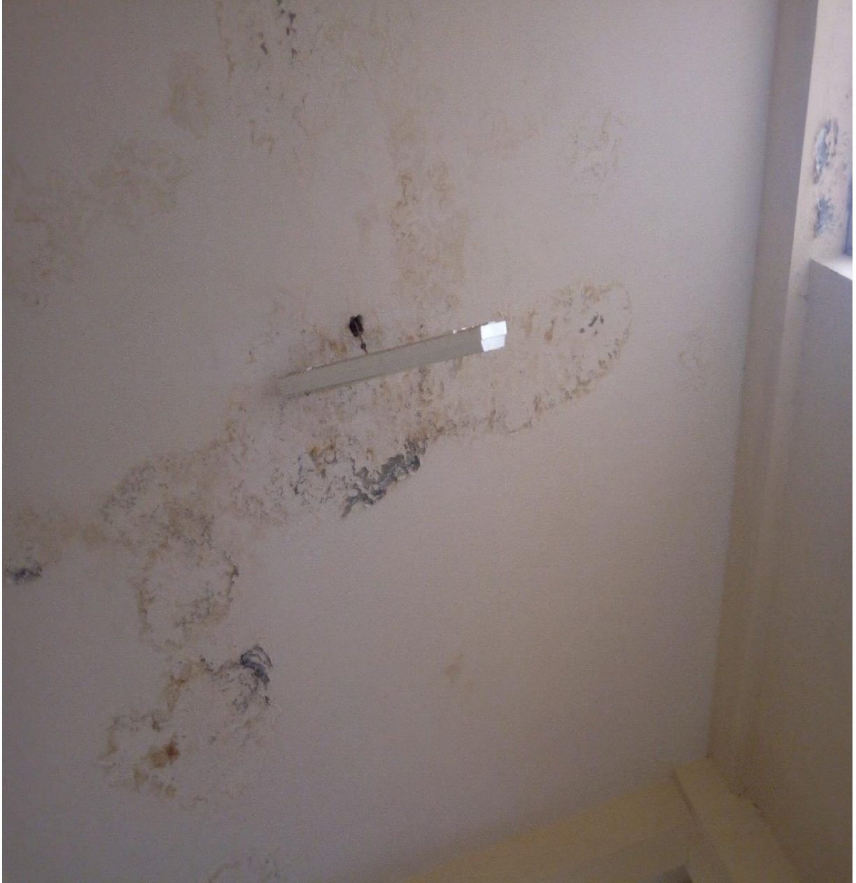
Figure D1.1 Leakage observed under side of slab on Dilla admin. Building (Image taken by researcher).
