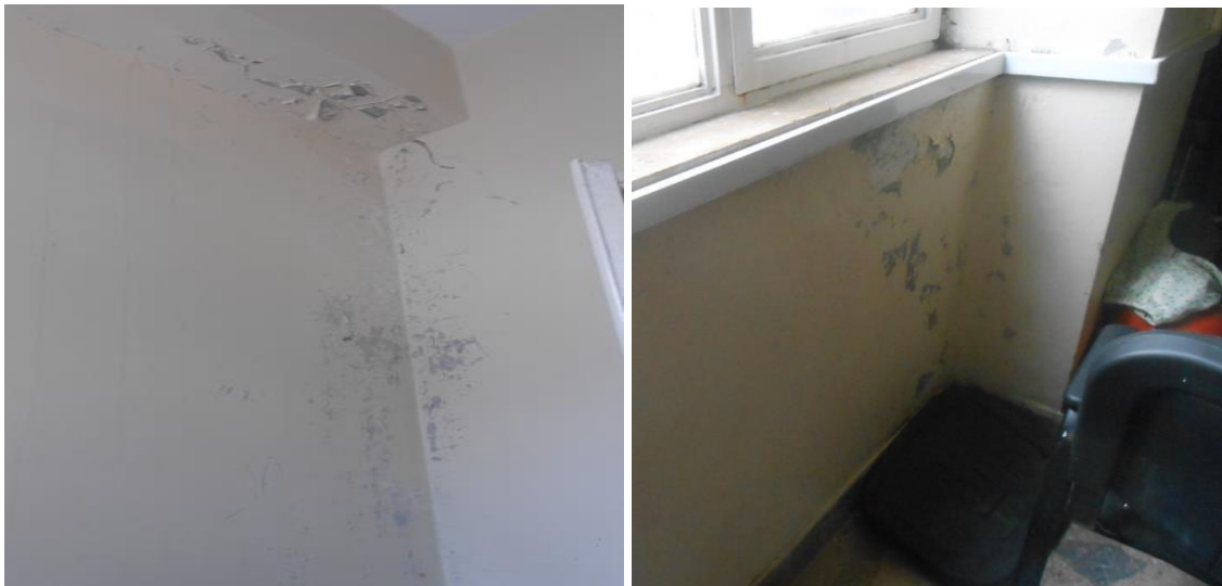
Figure 4.15 Internal dampness in ethio-telecom building in Hawassa (pictures taken by researcher).
