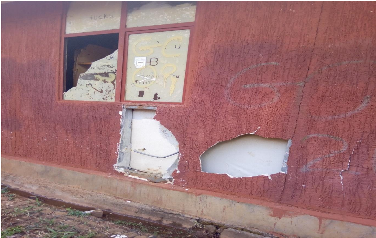
Fig D1.10. Temporary shelter deterioration in Dilla hospital building (Image taken by researcher).
