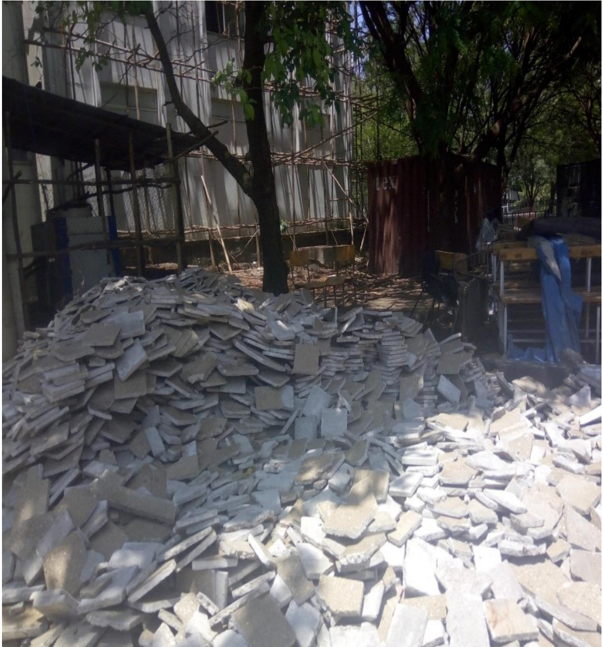
Figure D1.12. Maintenance work in Hawassa referral hospital building (Image taken by researcher).
