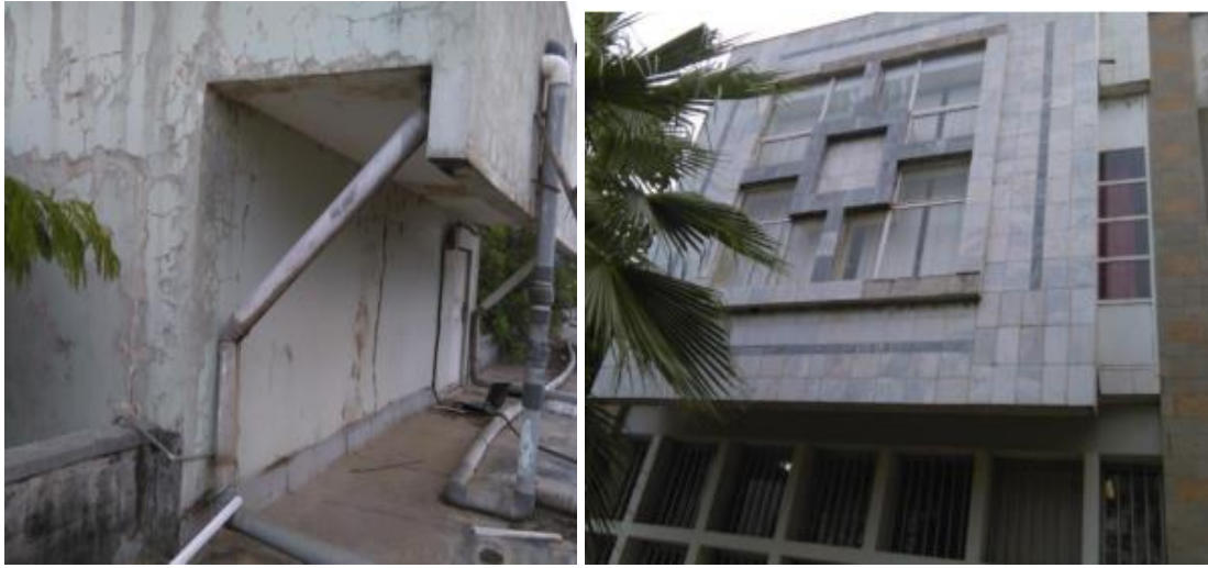
Figure 4.14 Damaged plastered and fallen off marble cladding at referral building (pictures taken by researcher).
