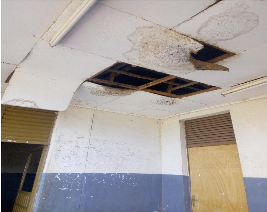
Figure 2.3 Ceiling deterioration by leakage through Ega in Dilla management building (image taken by the researcher).
