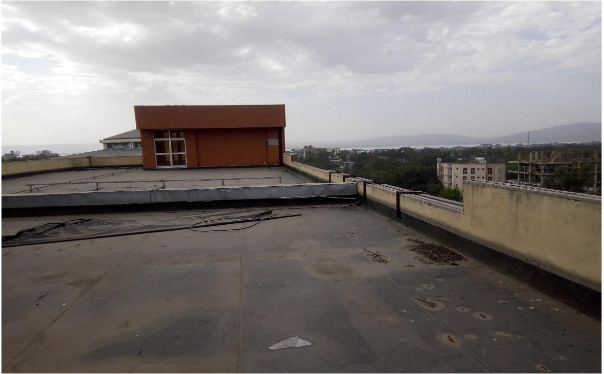
Figure D1.2. Damaged water proofing material in Ethio- telecom building Hawassa. Image taken by researcher).
