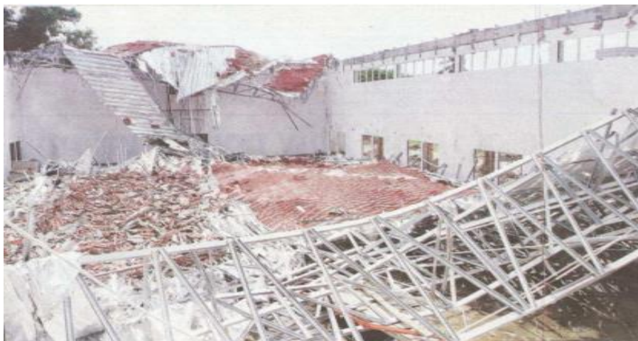
Figure 2.2 Roof structure collapsed in Kuantan (NST, 2005)
