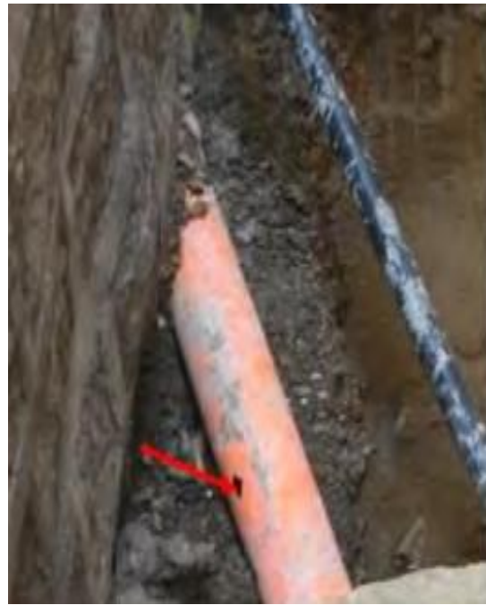
Figure 2.5 Leakage due to broken sanitary sewer (Yebichaye, 2016)
