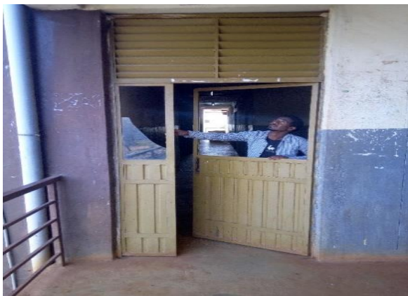
Figure 4.16 Broken doors, hinges, latch/lock (picture taken by researcher).
