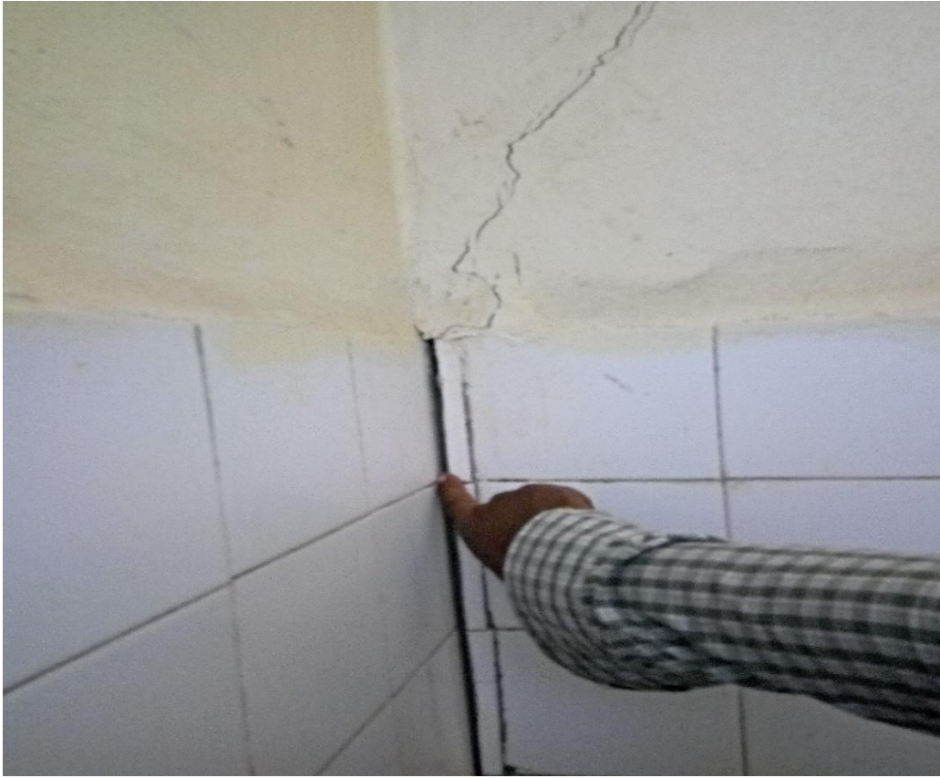
Figure D1.8. Displacement of wall observed on Arba Minch ethio-fishery apartment (Image taken by researcher).
