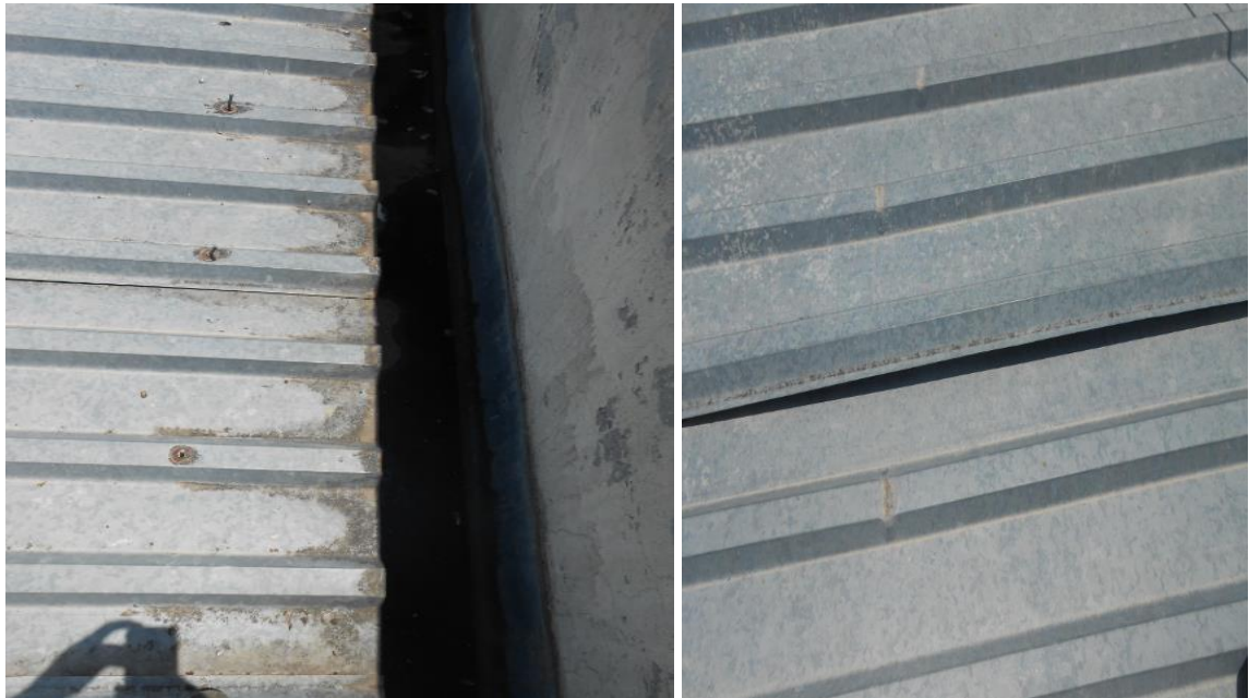
Figure 4.11 Damaged EGA roof cover at inpatient block in Hawassa referral hospital building (pictures taken by researcher).
