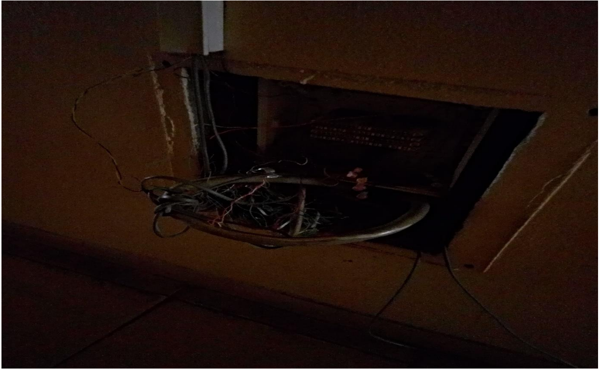
Figure D1.4. Uncovered switch board on Hawassa University School building (Image taken by researcher).
