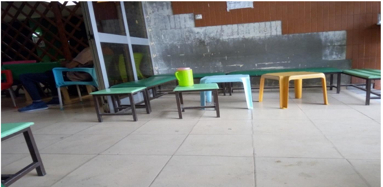
Figure D1.3. Peeling of wall clinker in Ethio-telecom building Hawassa. (Image taken by researcher).
