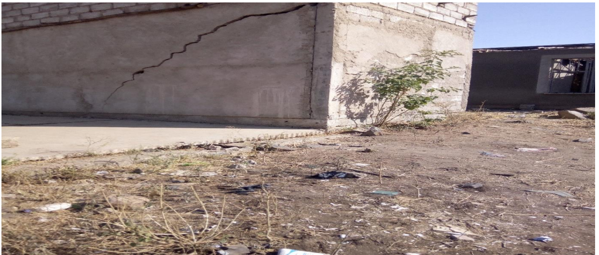
Figure D1. 7. Crack observed on Arba Minch referral hospital (Image taken by researcher).
