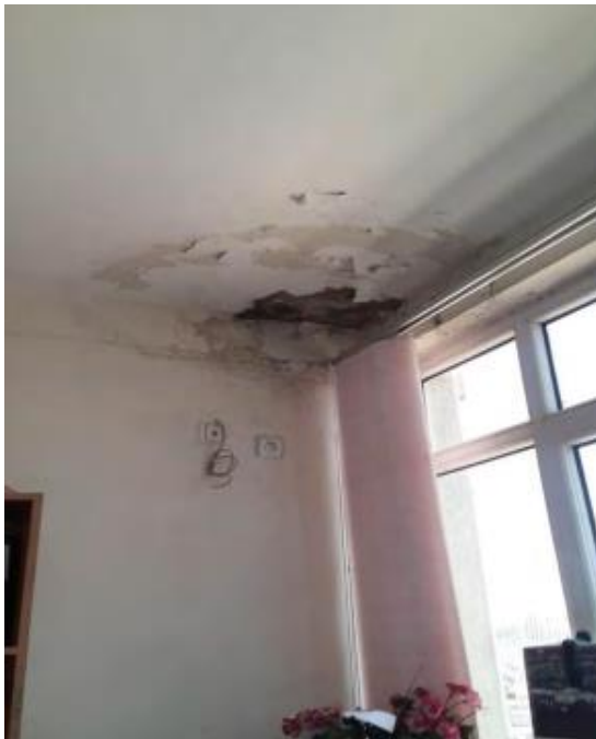
Figure 2.4 Ceiling leakage (Bedru M. , 2015)
