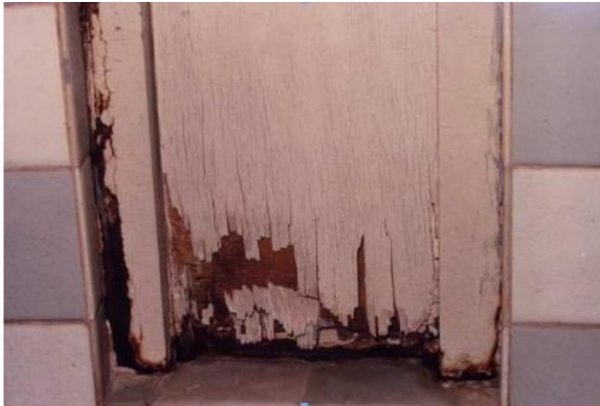
Figure 2.6 Rotting door due to moisture penetration effect (James & Ransom, 2006)
