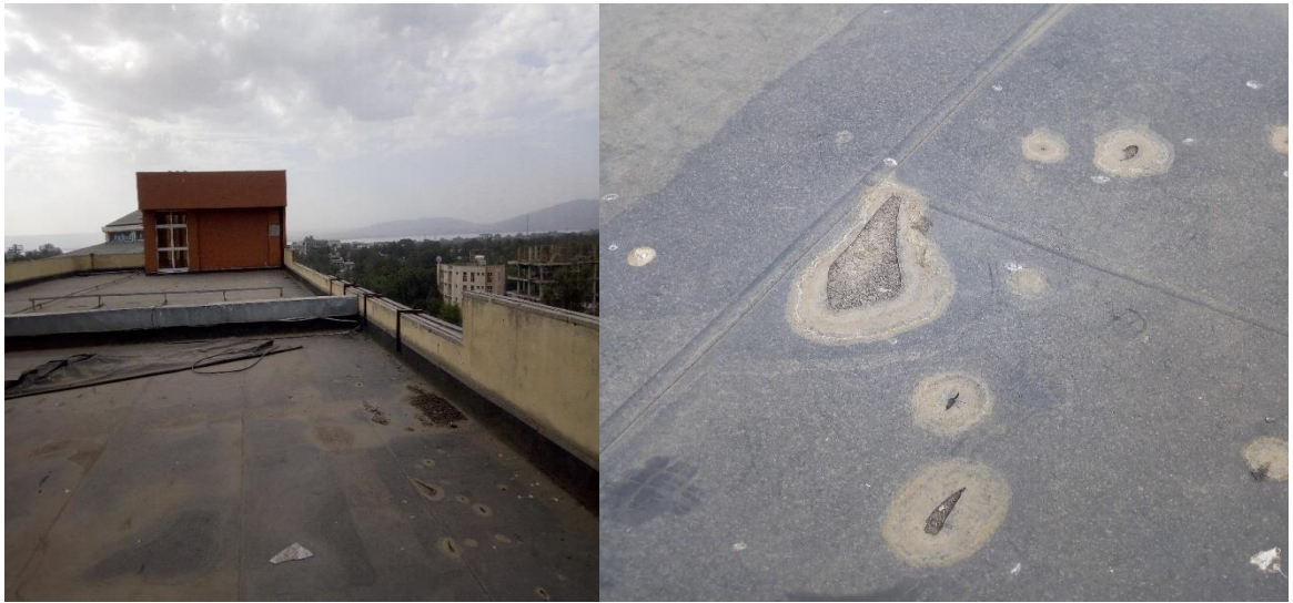
Figure 4.8 Damaged damp proof membrane on concrete slab roof in ethio-telecom building in Hawassa (Image taken by researcher).
