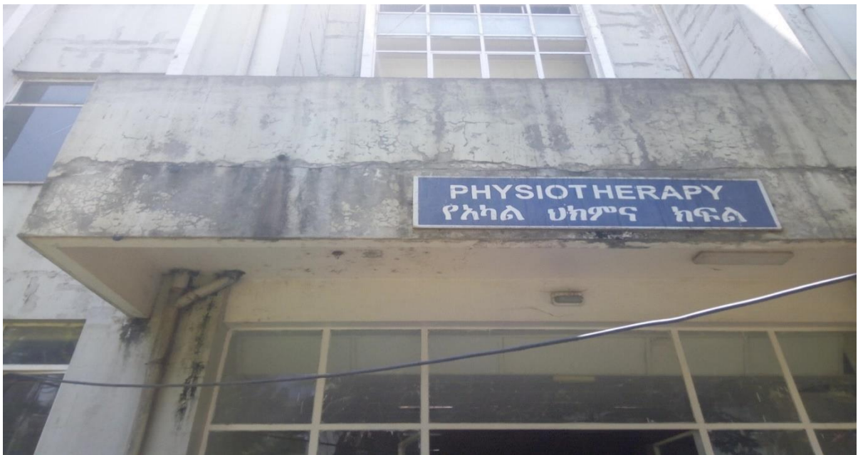
Figure D1.11. Hawassa Referral hospital peeling of painting, fissure cracks (Image taken by researcher).
