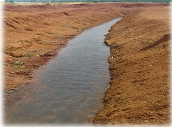
Canal sides were eroded
