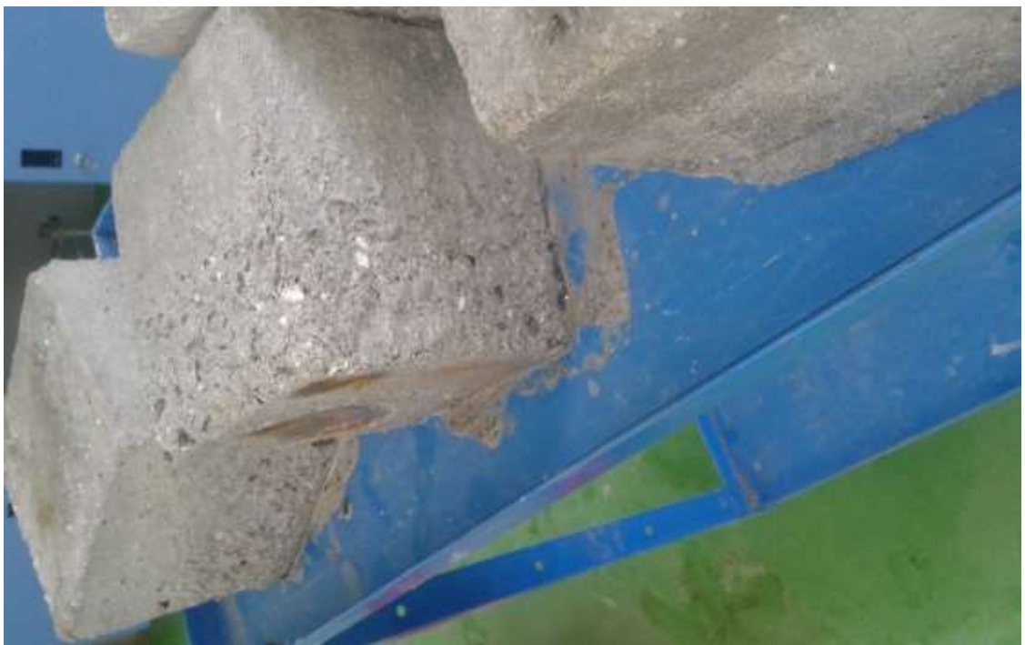
Figure B. 2 Deterioration due to Sulphuric acid attack
