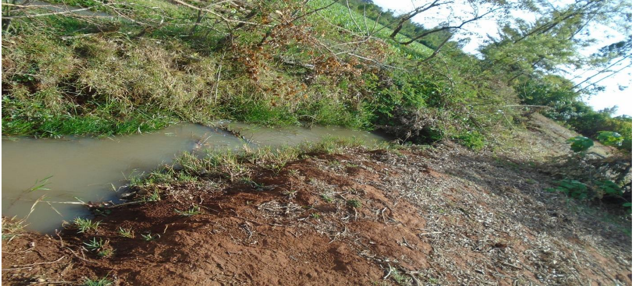
Figure 5: Canal siltation, and grass and weed growth problem at Ella
