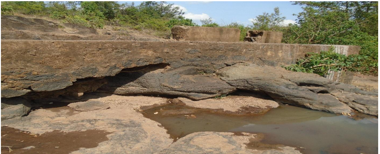
Figure 4: Downstream scouring problem at Bossa scheme
