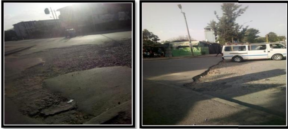
Figure 4-18: chronic pavement distress in the route old bus station to old market. (Source: Girma Yane)
