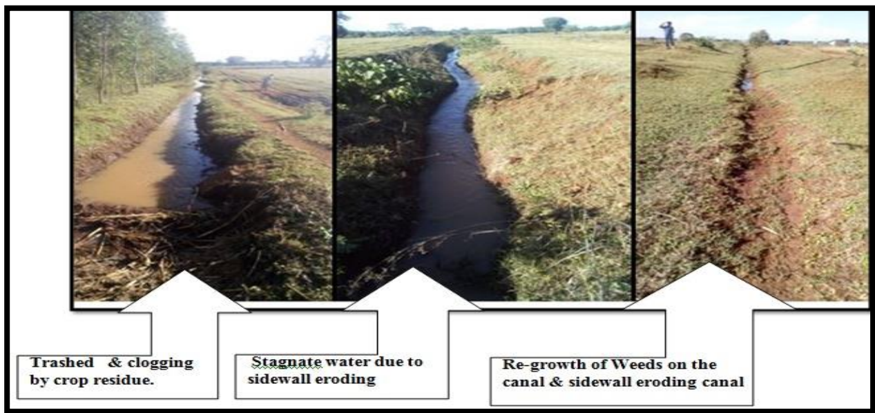
Figure 4.1:-Poor canal maintenance
