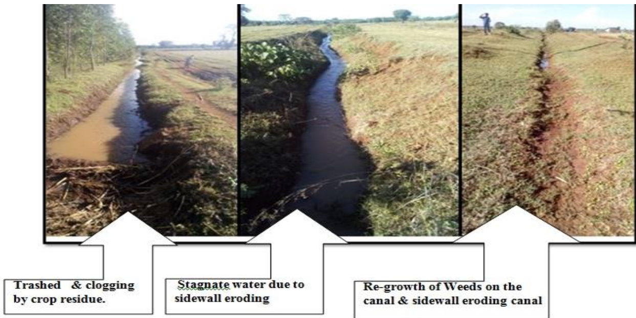
Appendix figure 3. Poor canal maintenance
