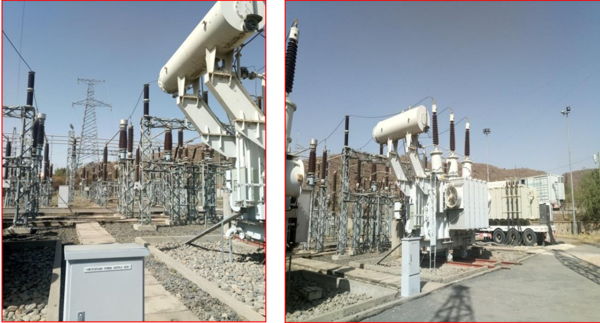
Figure 1. 2: Overview of Yirgalem substation [2]. (Source: on-site visit)
