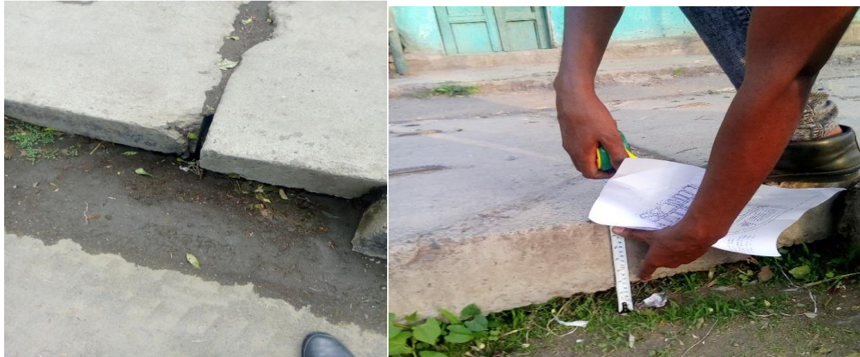
Figure 4.15: Manhole opening closed by garbage and less depth of opening
