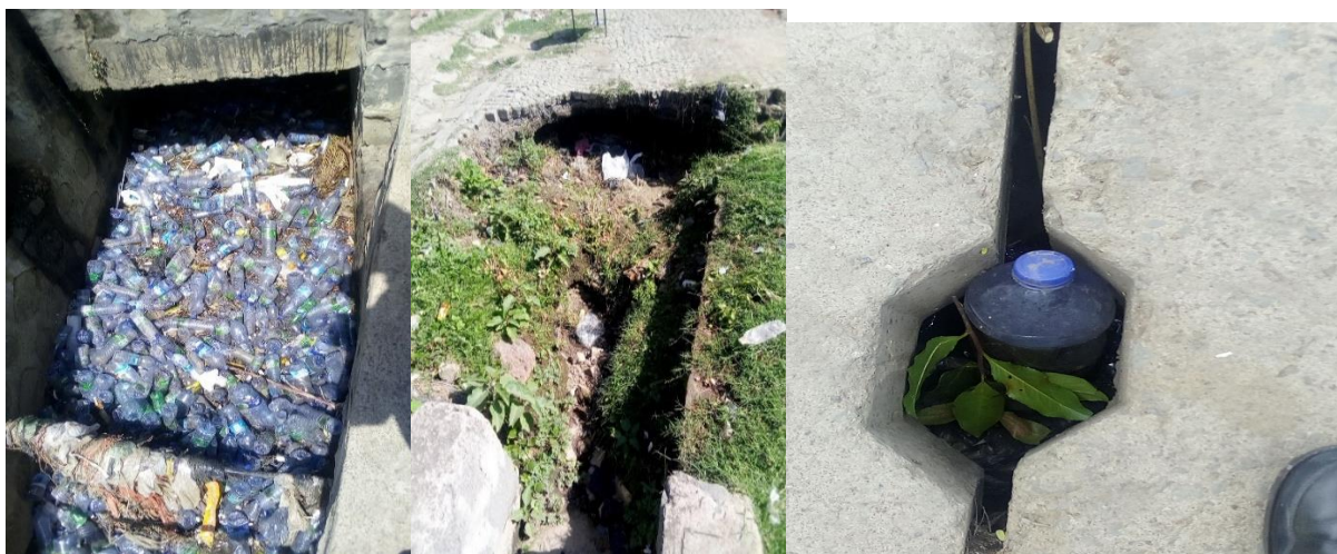
Figure 4.14: Blocked closed canal (right side), Blocked open canal (left side) and Damaged canal (middle)
