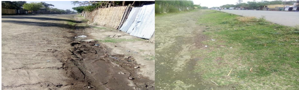
Figure 4.13: Effect of neglecting collector Drainage Systems around Lenda Ber(left side) and Mahal Arada (right side)
