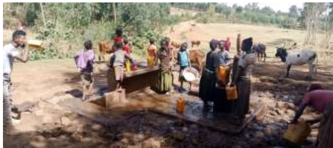
Figure: Broken down of spring pipe line
