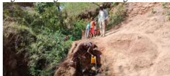
Figure: Broken down of spring pipe line
