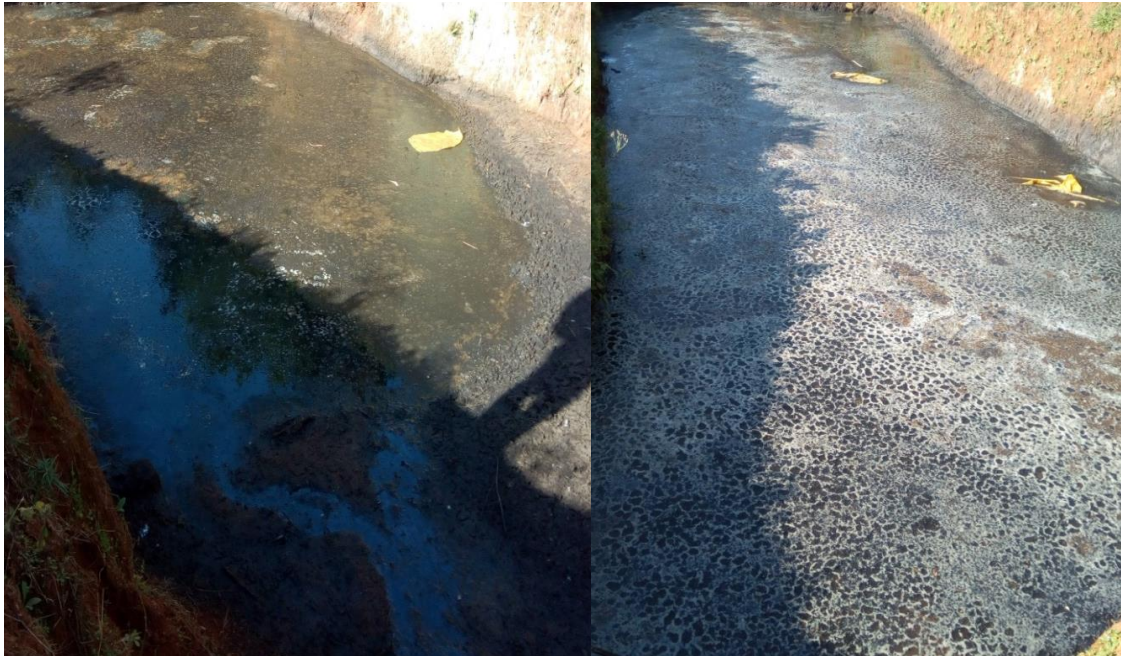
Figure a 3: Improperly constructed disposal pits and its discharge into receiving environment
