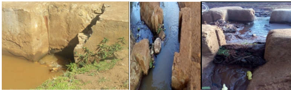
Fig-7, Absence of water control gates in the Ela scheme
