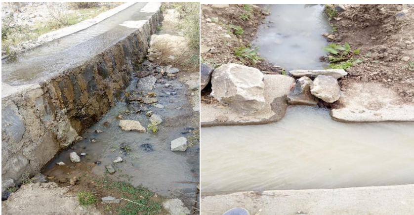
Figure 4. 3:Overtopping of water on main canal and water control by traditional manner
