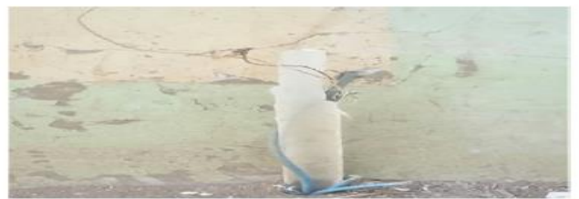
Damaged schoolnet Network cable
