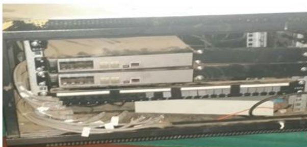
Damaged Non POE Switch
