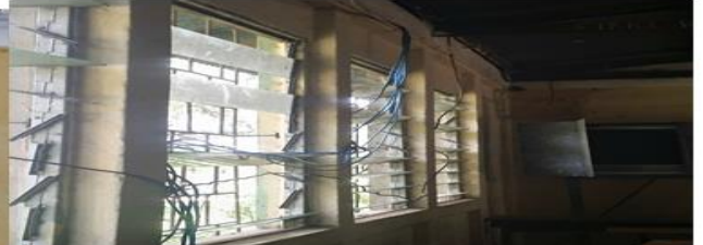
Damaged Plasma Tv network cable
