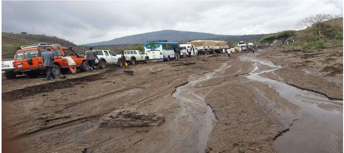
Figure 1.2: Thick silt deposit overlay on pavement resulting from flood blocked the traffic (Photo by Author; August 24, 2017)
