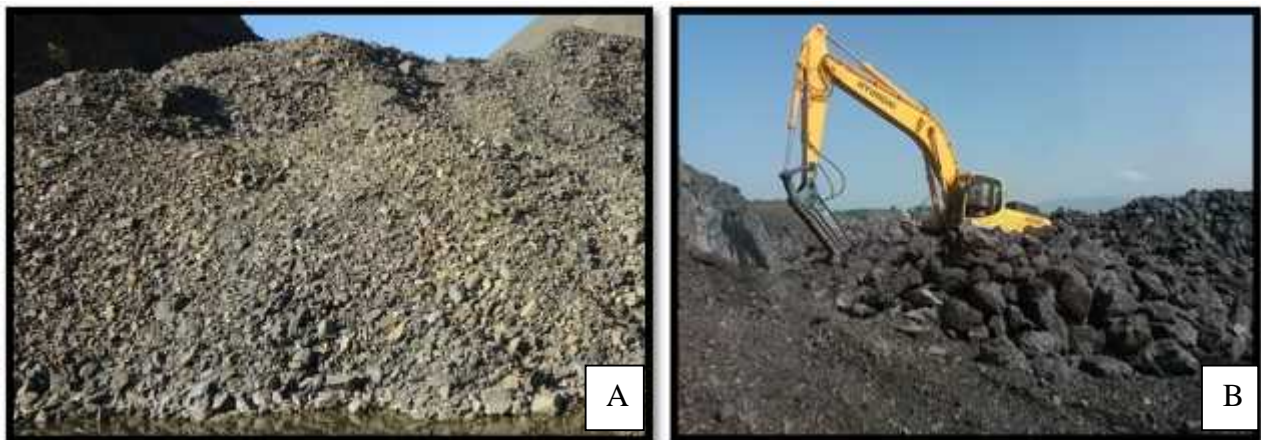
Photo 3-1 : Material production at Ribb dam project (A) slightly weathered fine rock (B) blasted rock
