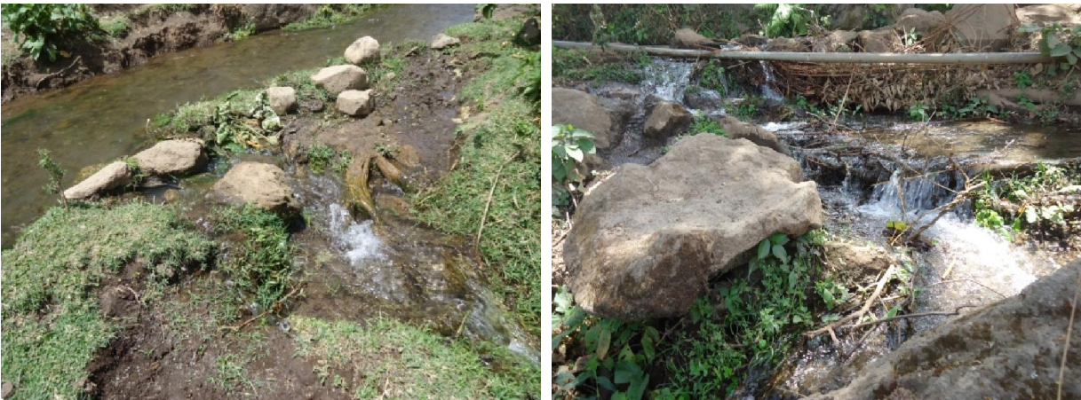
Figure 7: Loss of water due to canal breaking on secondary canal
