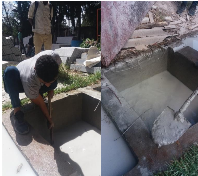
Figure A 1: Granite sludge in reservoir tank
